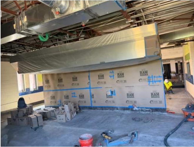
2026.07.14 – New kitchen exhaust hood
