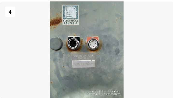
400Amp contactor for F2 & F4 (East side of field) labeled A2 & A4
