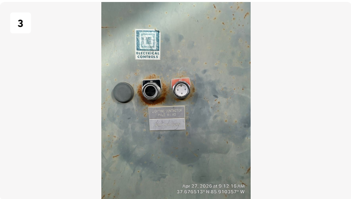
400Amp contactor for F1 & F3 (West side of field) labeled A1 & A3
