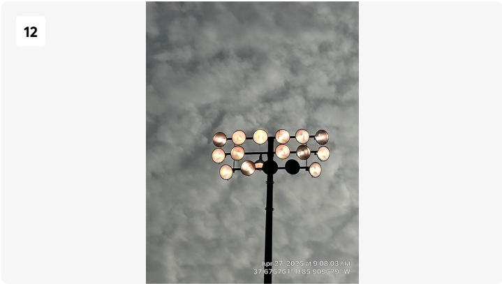
Closeup of F3 Pole, 2 outages, 1 hanging fixture, 14 pink lamps
