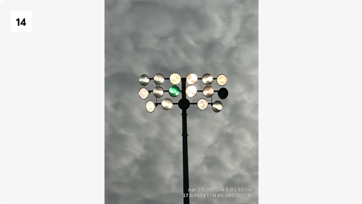
Closeup of F4 Pole, 2 outages, 1 green lamp, 3-4 pink lamps, and a few dim fixtures
