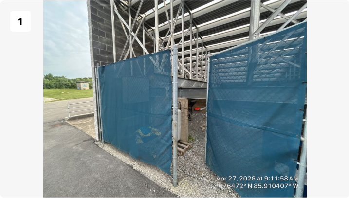
Access to contactors under West bleachers
