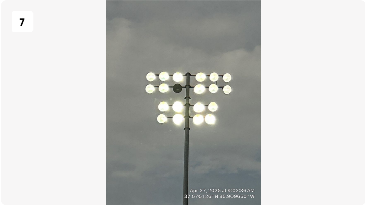
Closeup of F1 Pole, 1 outage
