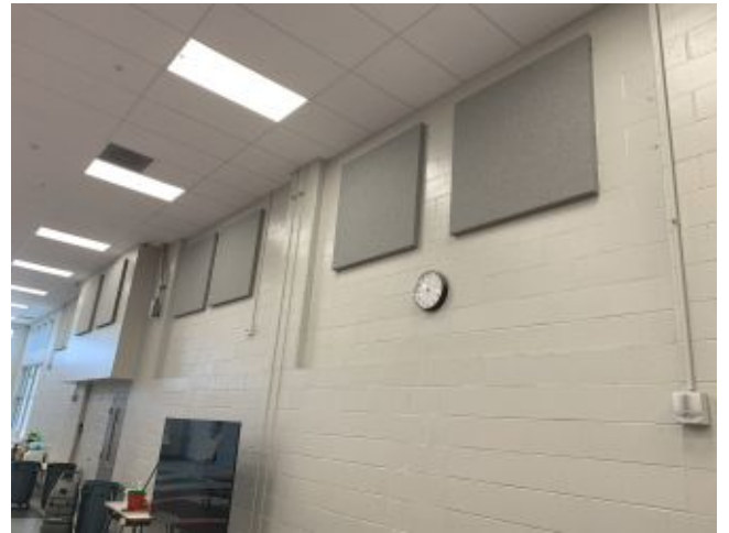
2026.05.28 – Acoustic panels in cafeteria
