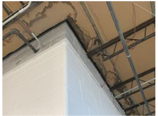
2026.06.04 – Water damage in Classroom #202
