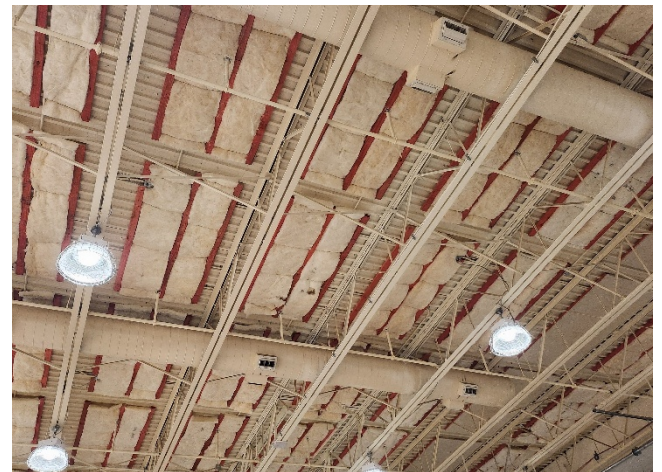
2026.04.14 – Furring strips and batt insulation on ceiling of gymnasium for new acoustic panels
