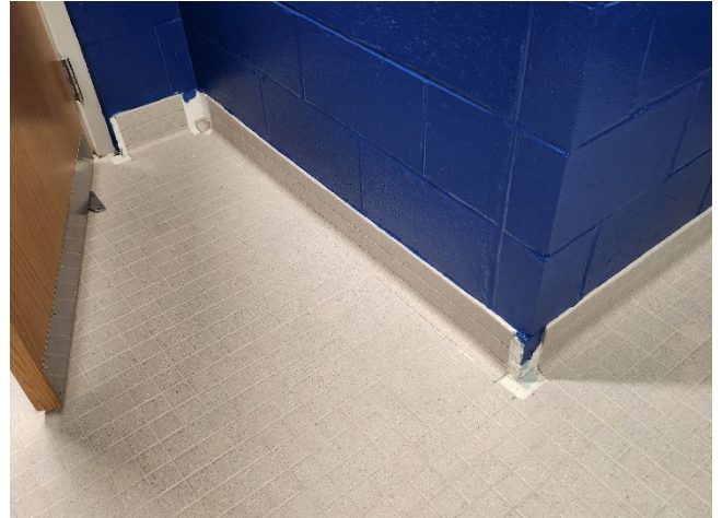
2026.03.12 – Missing tile corners in Group B Restrooms
