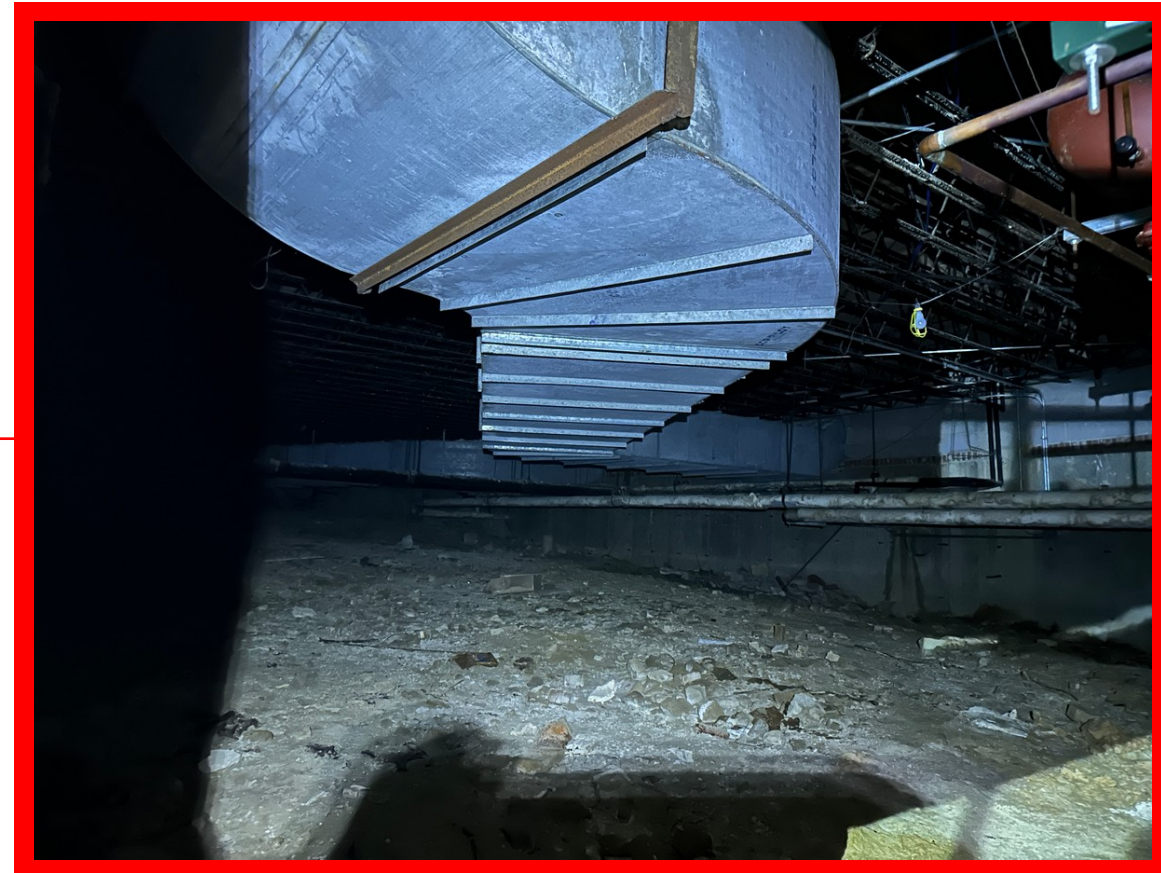
PHOTO OF UNDER STAGE RA DUCTWORK.
