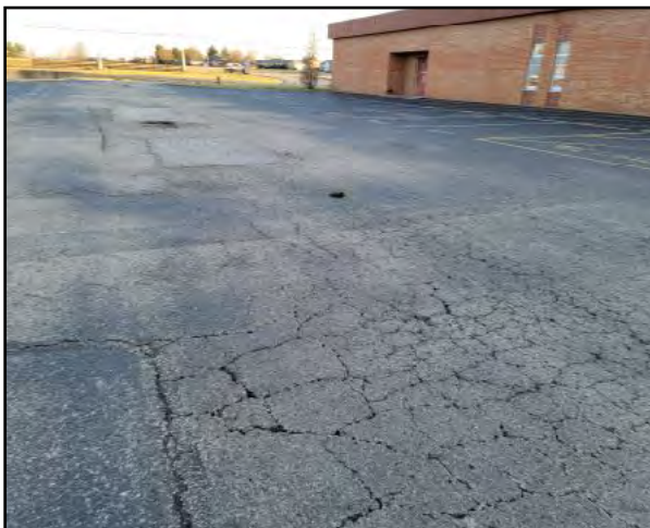
Photo 3. View of cracking in asphalt pavement.
