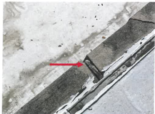
Concrete coping joints are failing
