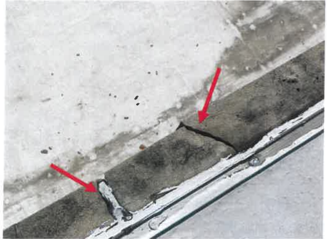
Another failing joint and large crack
