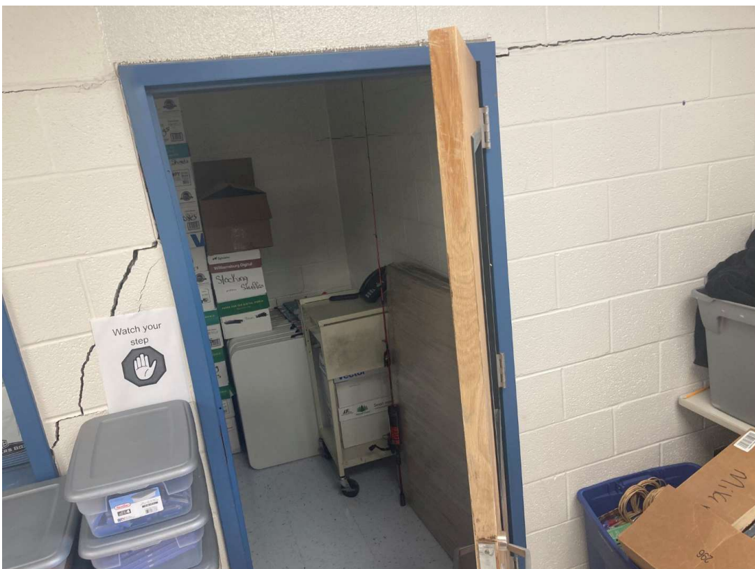
Displaced wall with significant cracking causing inoperability of door due to 'racked' frame.
