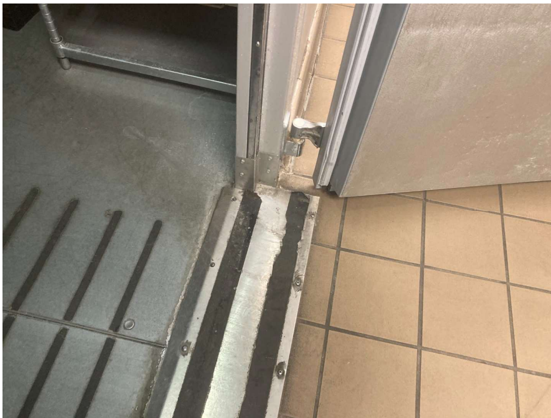
Damaged cooler/freezer box with misaligned doors, due to heaving floors and walls.
