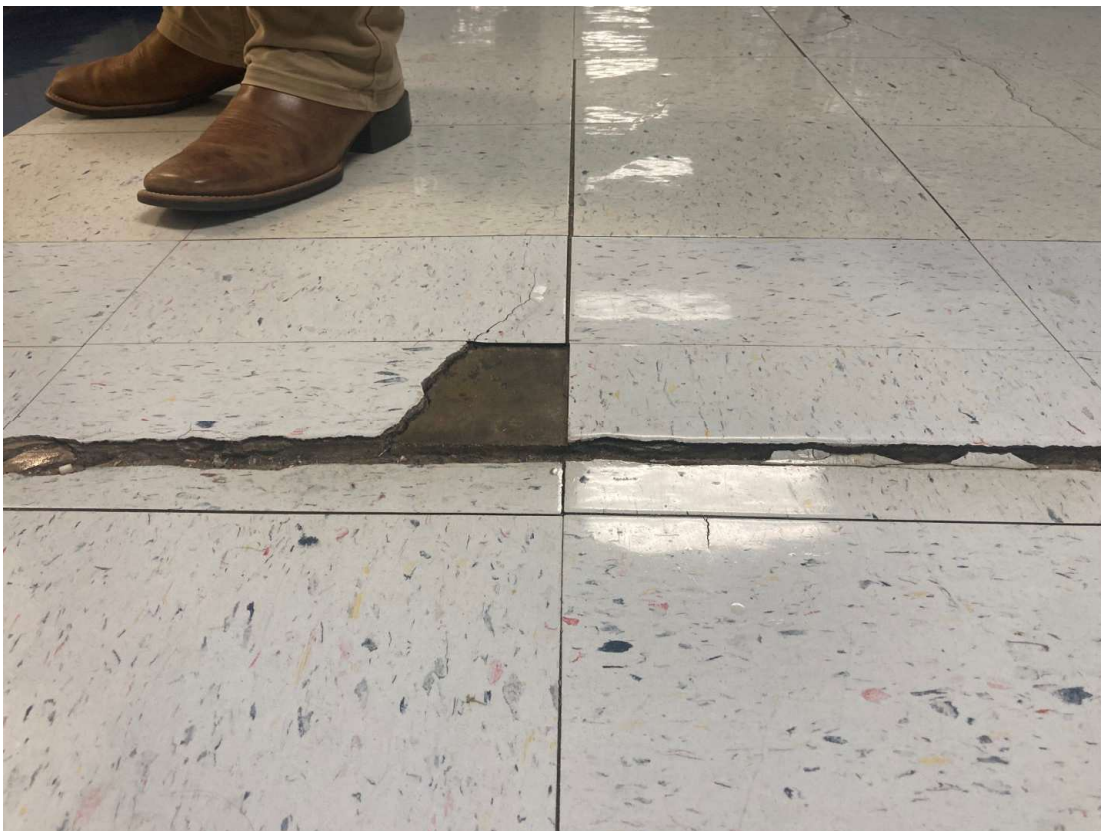
Vertical displacement of slab at primary classroom wing corridor causing tripping hazard and damaged flooring.
