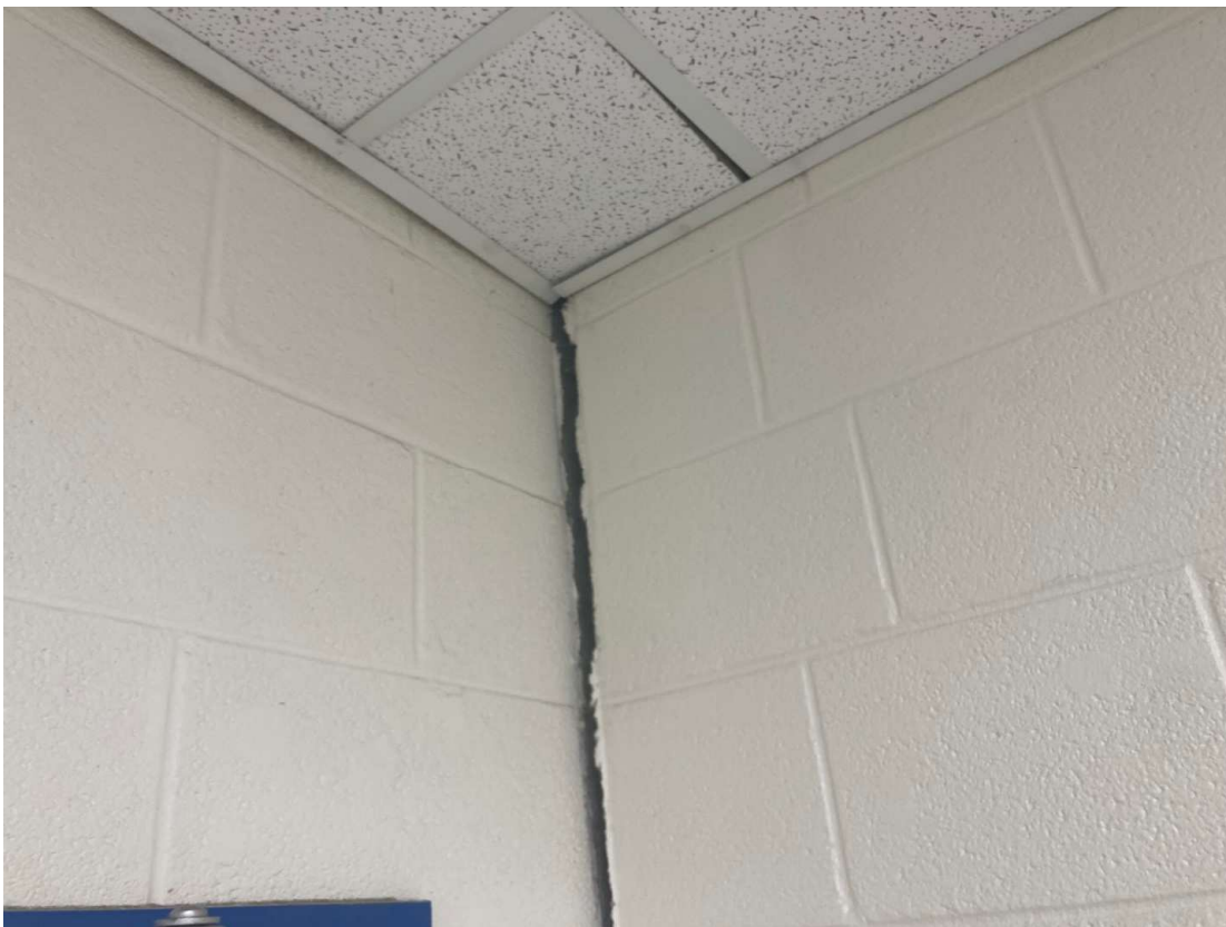
Separation of masonry walls and horizontal displacement of masonry walls, typical throughout building.
