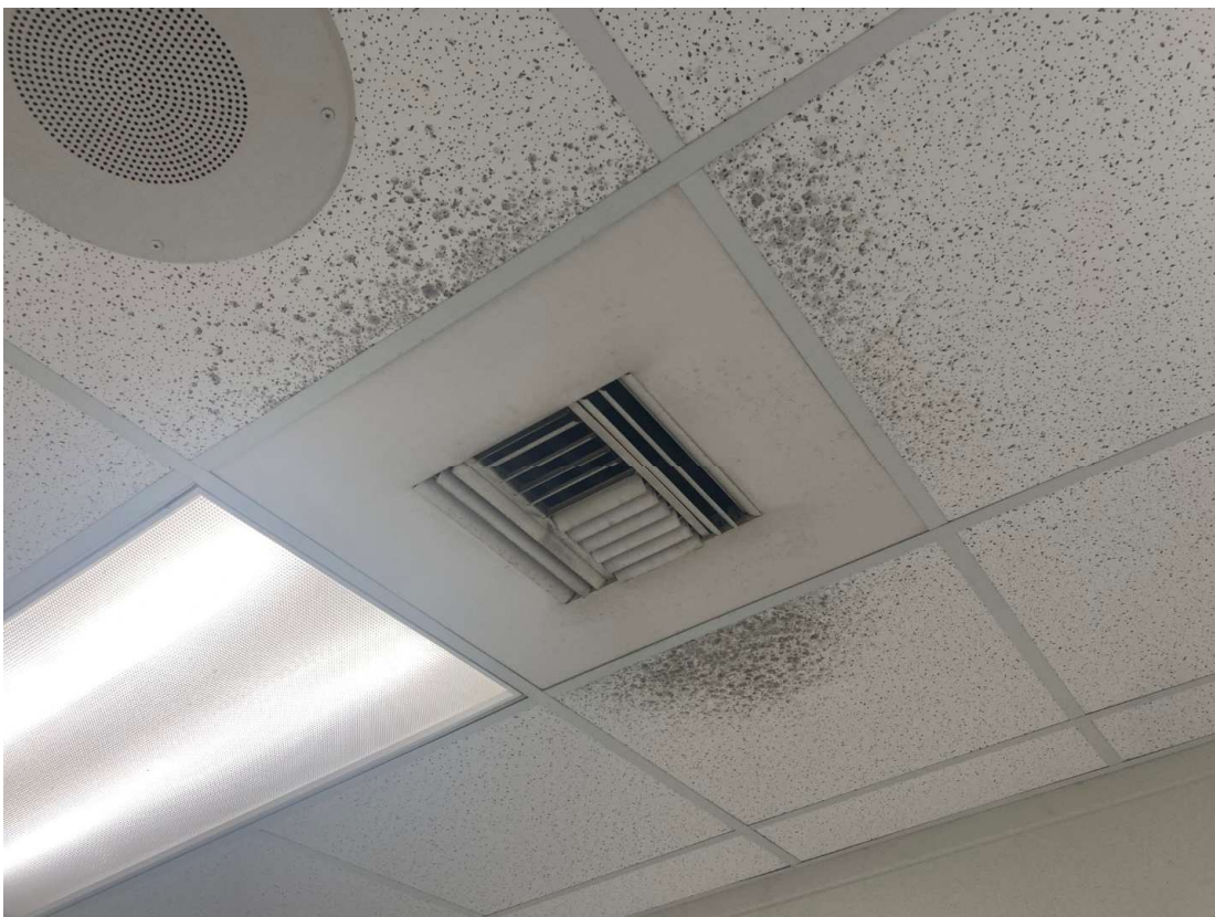
Abnormal organic growth on ceiling tile potentially due to air infiltration and damage to the duct.
