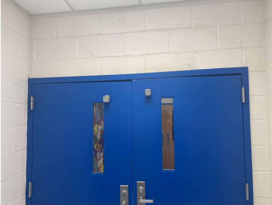
Interior frame and door that has 'racked' causing intermittent inoperability and ongoing maintenance.
