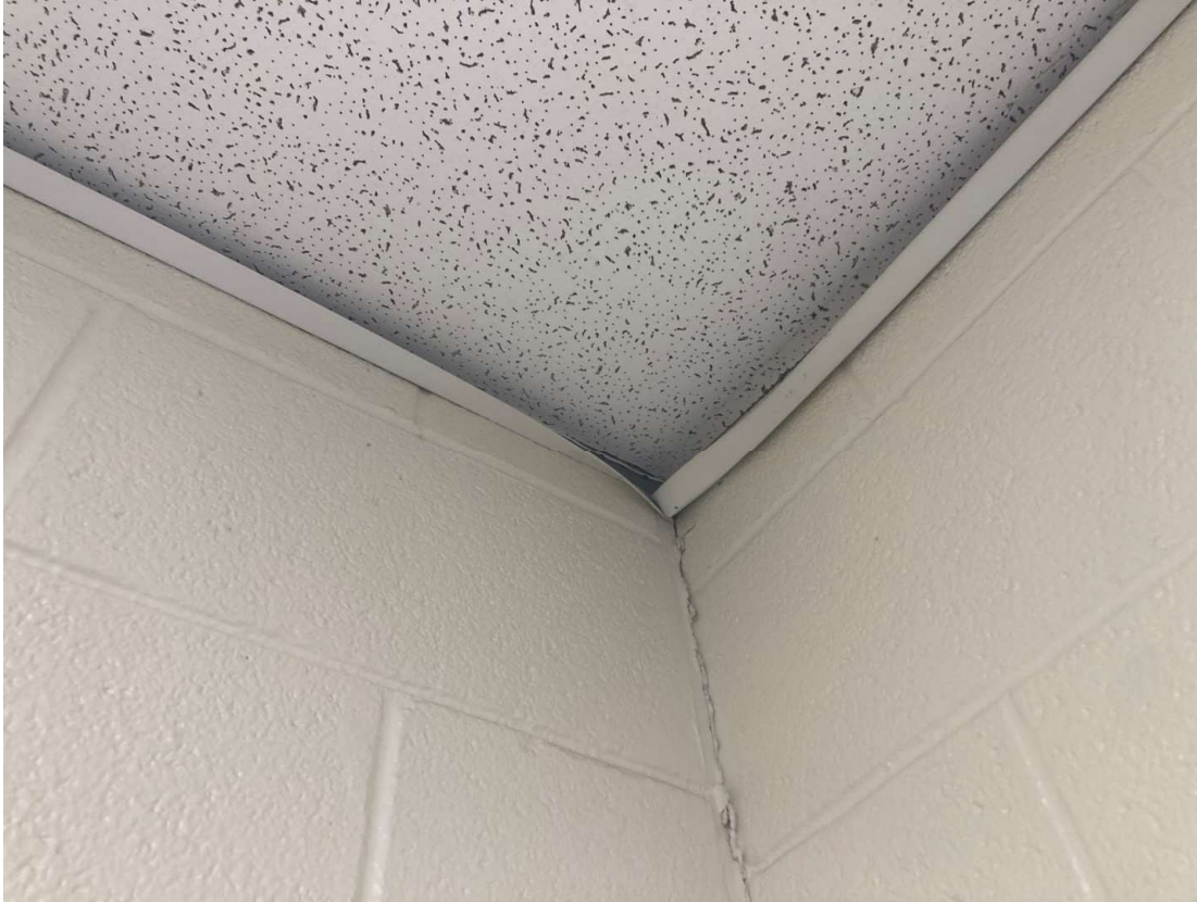
Vertical displacement of walls causing damage to interior finishes.
