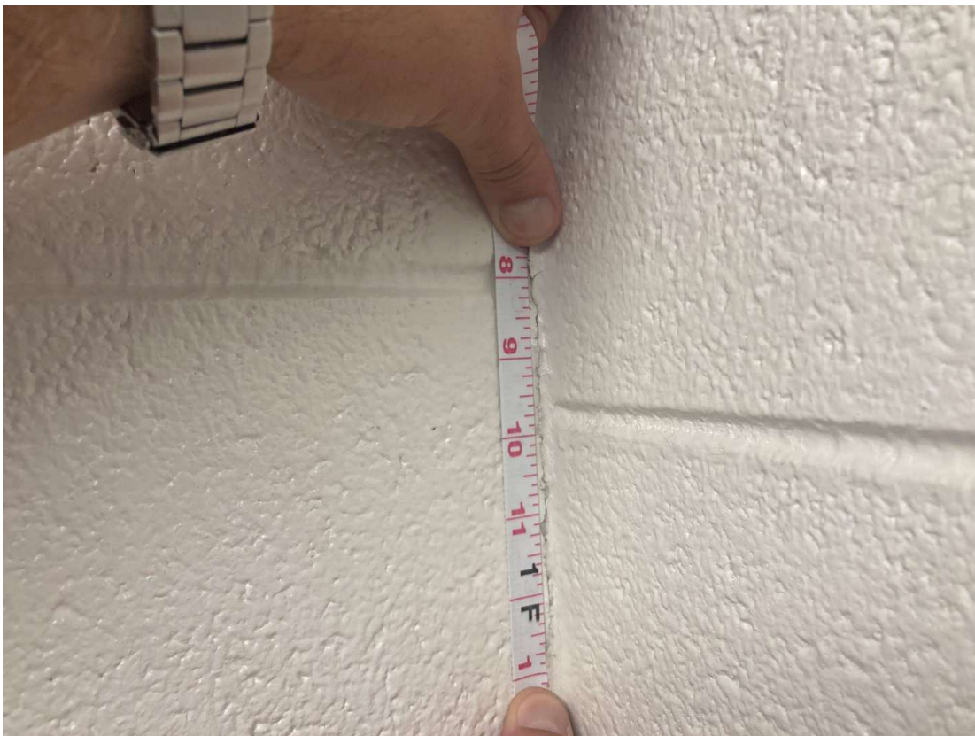
Vertical displacement of masonry walls as measured in inches. Note that the horizontal joints should align.
