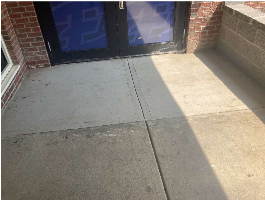
Exterior walk at egress door causing positive slope toward building and door.
