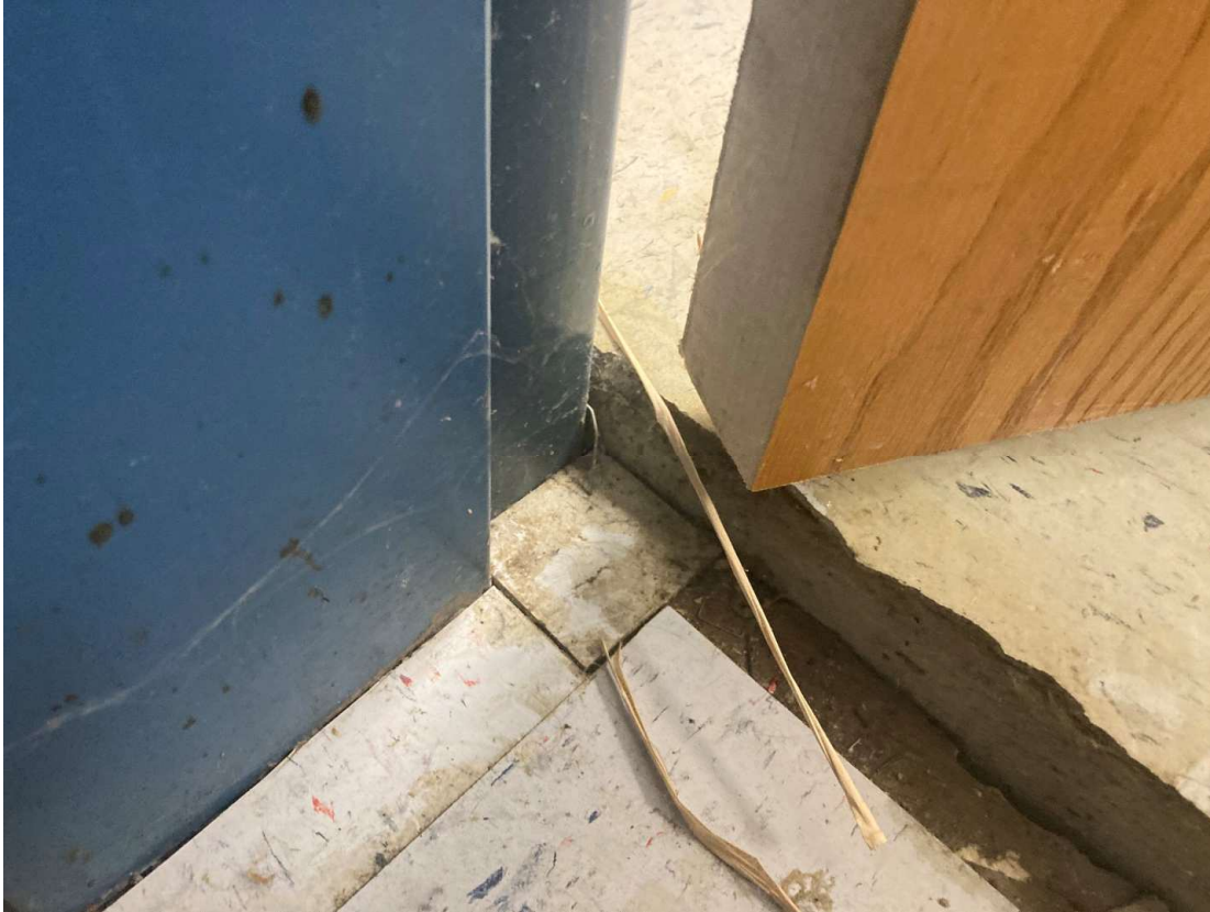
Vertical displacement of floor slab causing tripping hazard and inoperable door.
