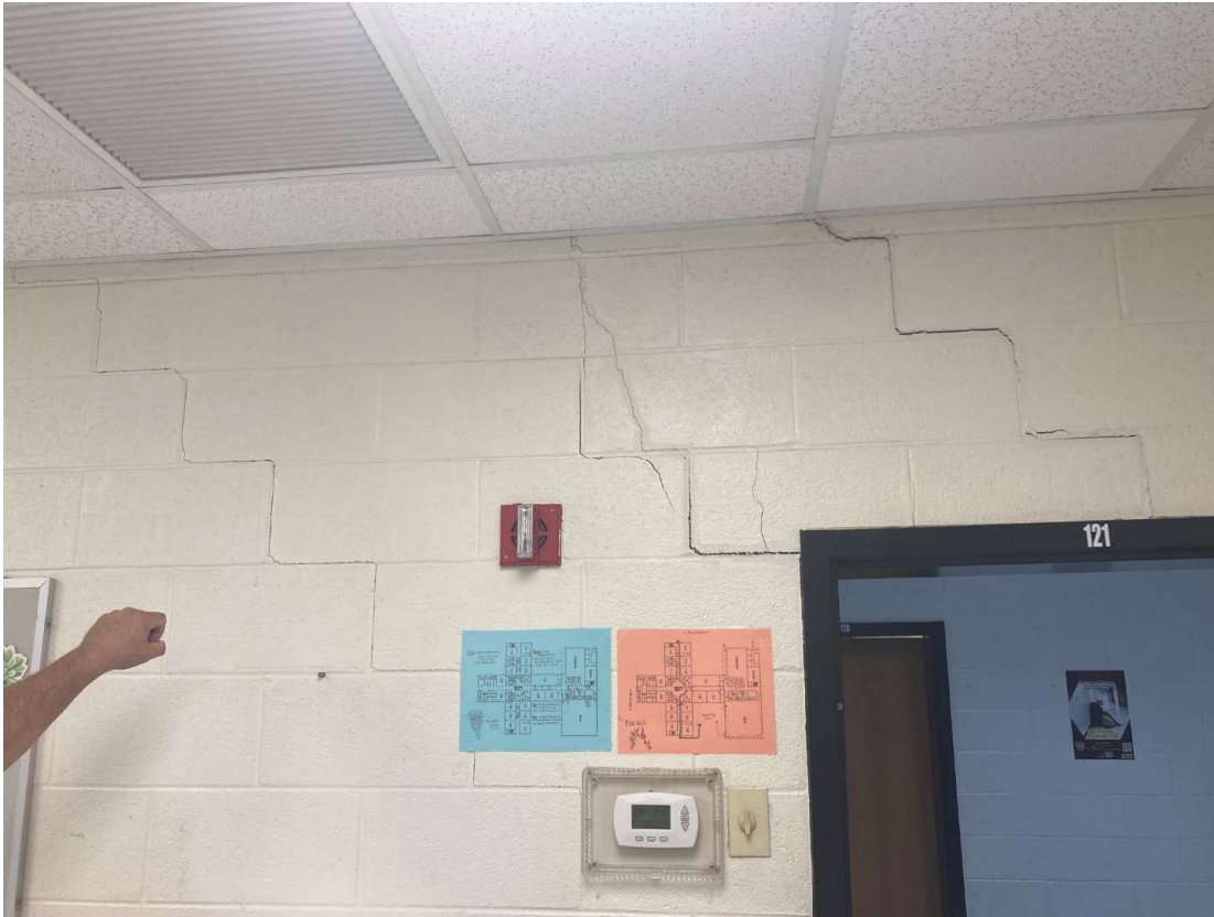
Cracked interior load-bearing CMU wall at corridor, typical throughout building.
