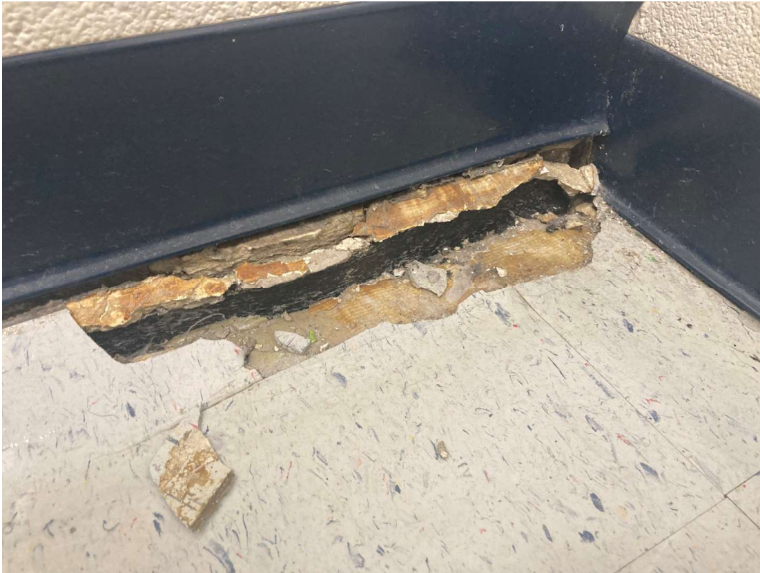
Vertical displacement of masonry walls causing a 'gap' at the floor and damage to interior finishes.
