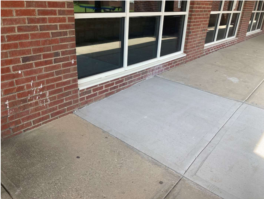
Exterior Sidewalk has heaved creating a tripping hazard.
