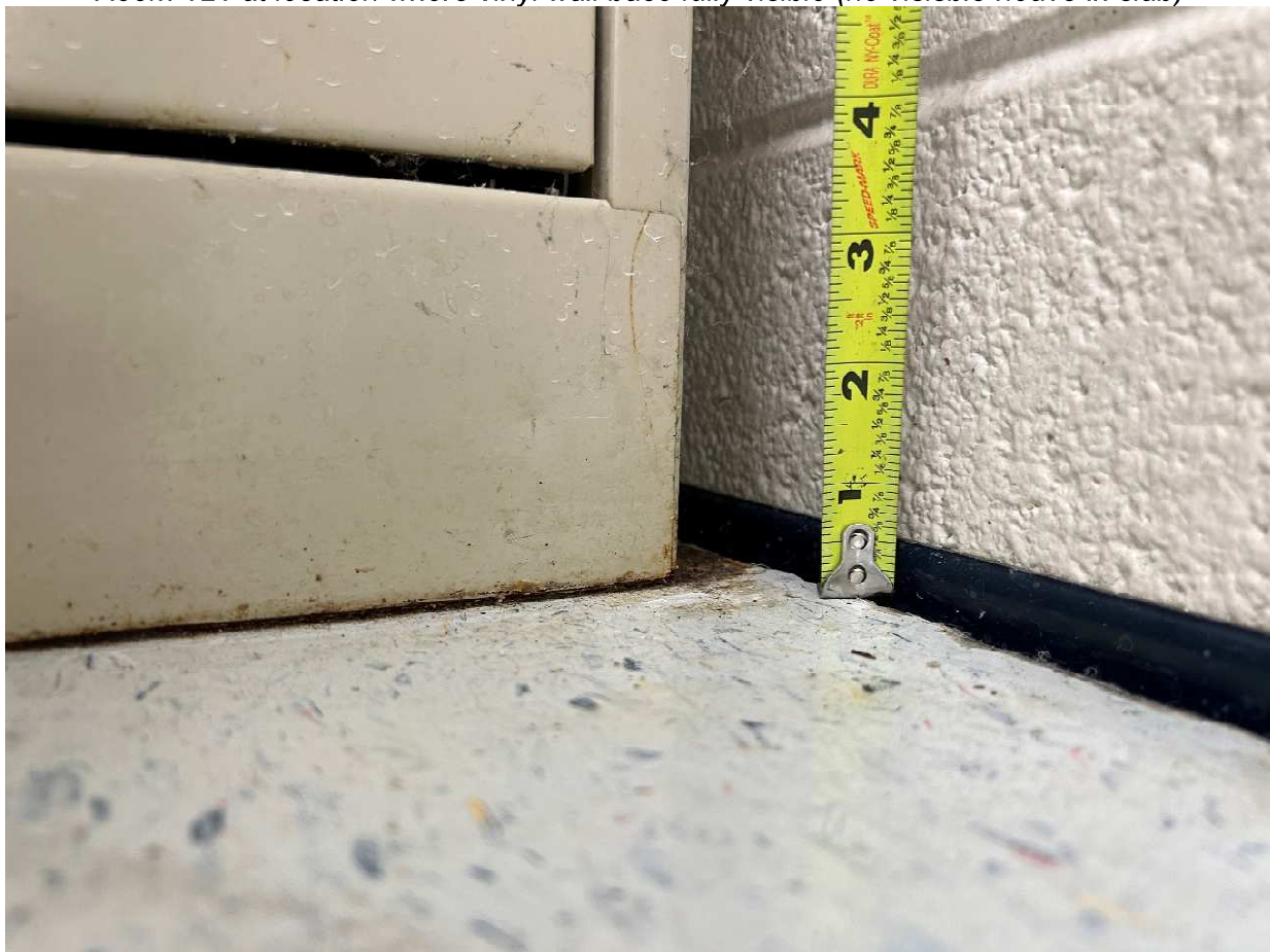
room 121 at slab location where heave is roughly 3 1/4" +/-.
