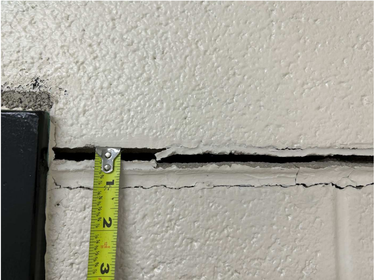
Room 121, closeup view of gap in CMU (measuring approx 3/8").
