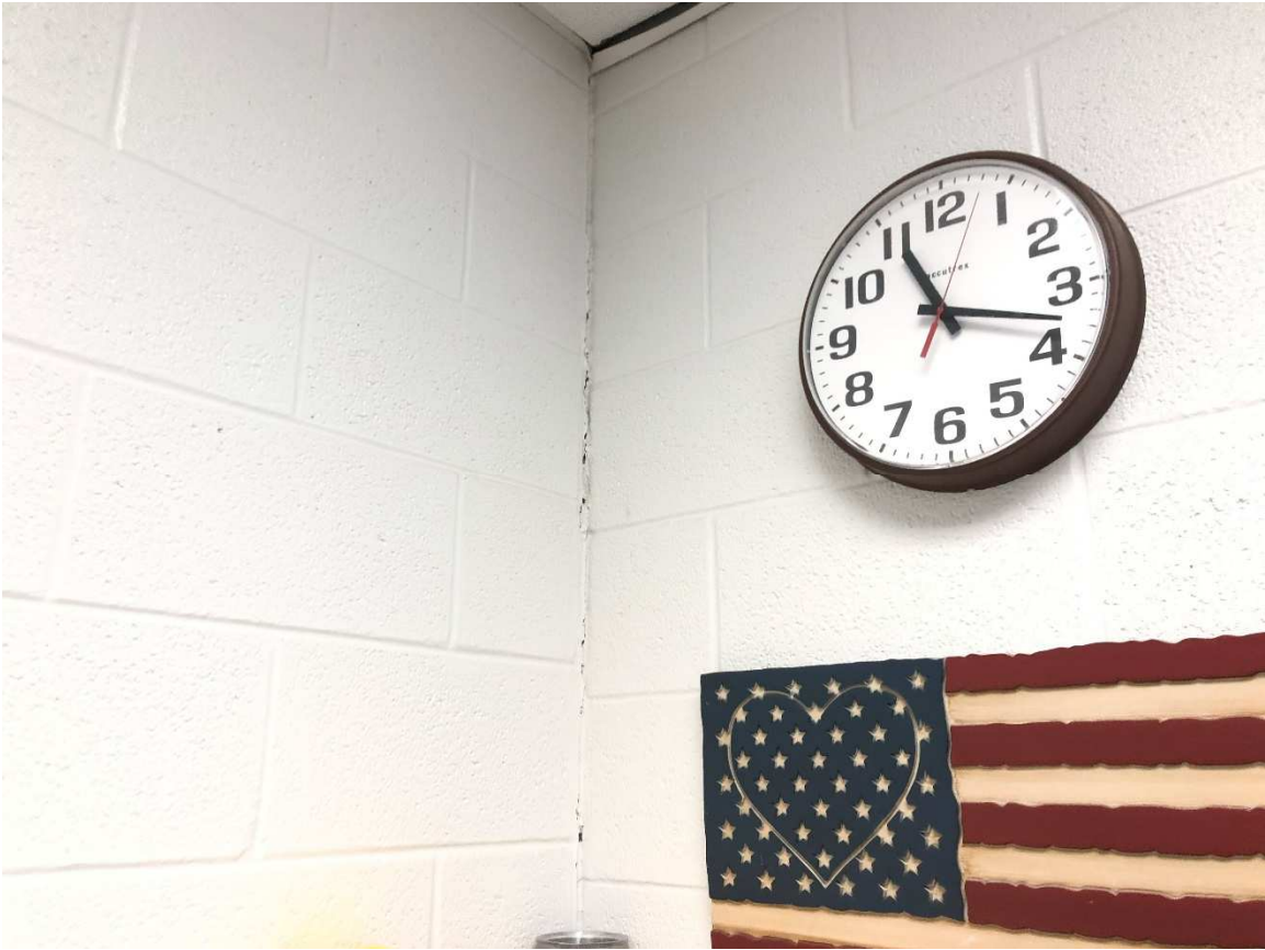
Interior partition heave
