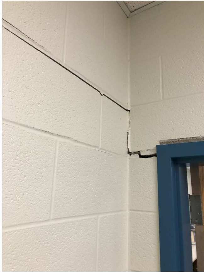
Significant crack in CMU wall
