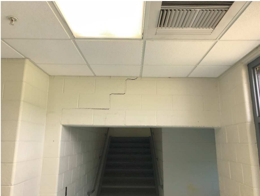
Heaving between jambs of steel lintel. Distortion of steel lintel and cracking of CMU has occurred.
