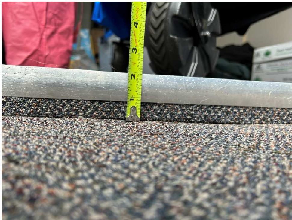
Visible heave in concrete slab near exterior door of youth service center, measuring approx 2".
