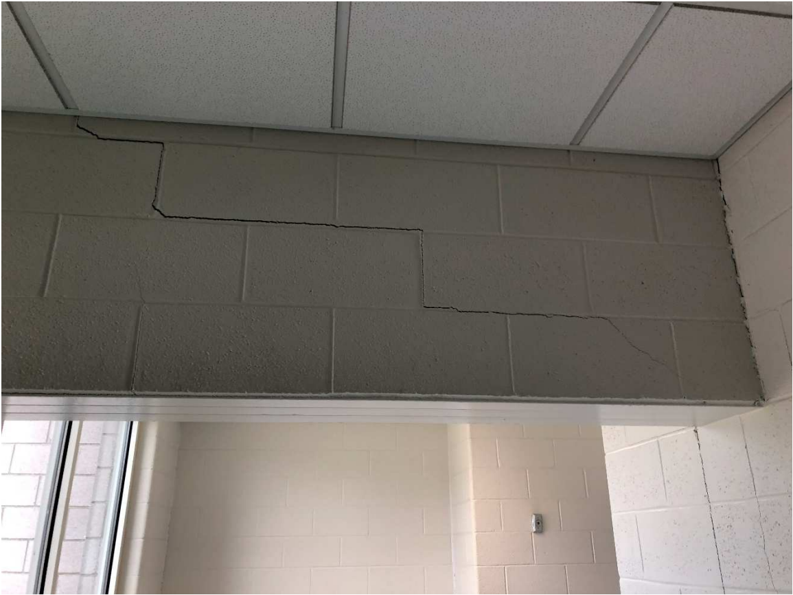
Stress cracks in CMU over heaving of steel lintel.
