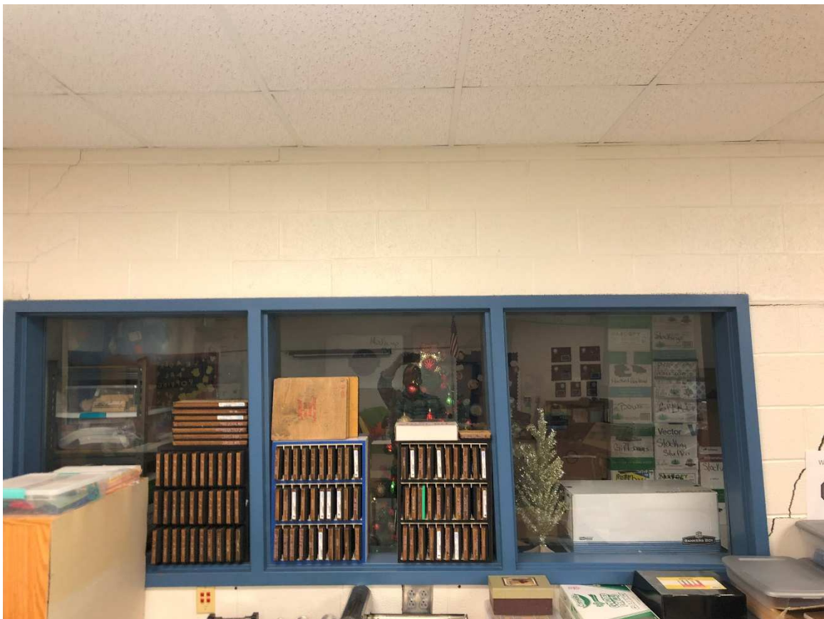
Cracking in partition wall. Window frame significantly out of level.
