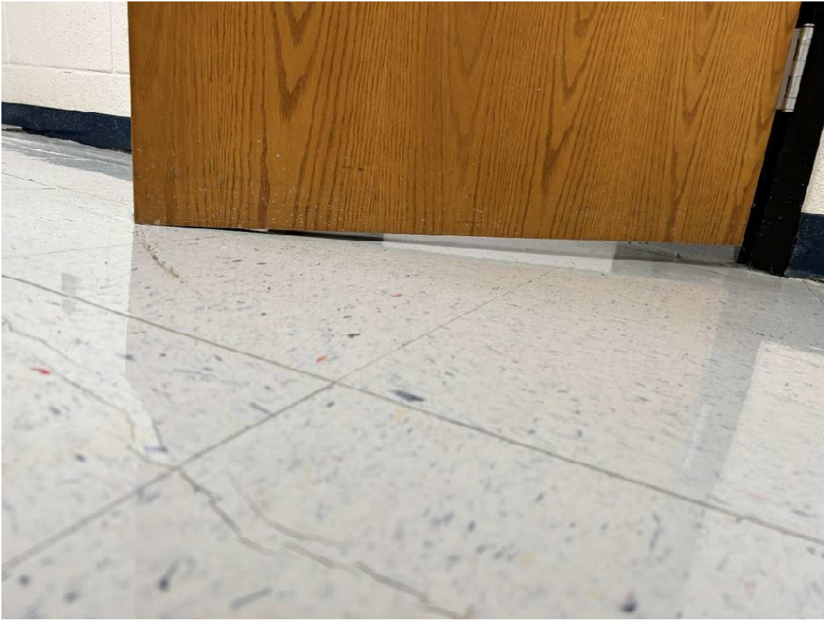
Gap under door displaying slope in floor elevation.
