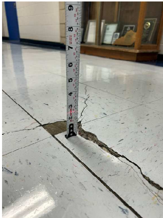
Laser level indicating a rise in concrete slab of approx. 5 1/4" from exterior door to most severe heave location in corridor.
