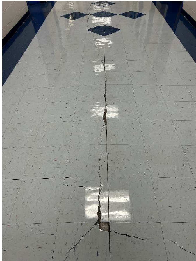
Heaving of slab on grade
