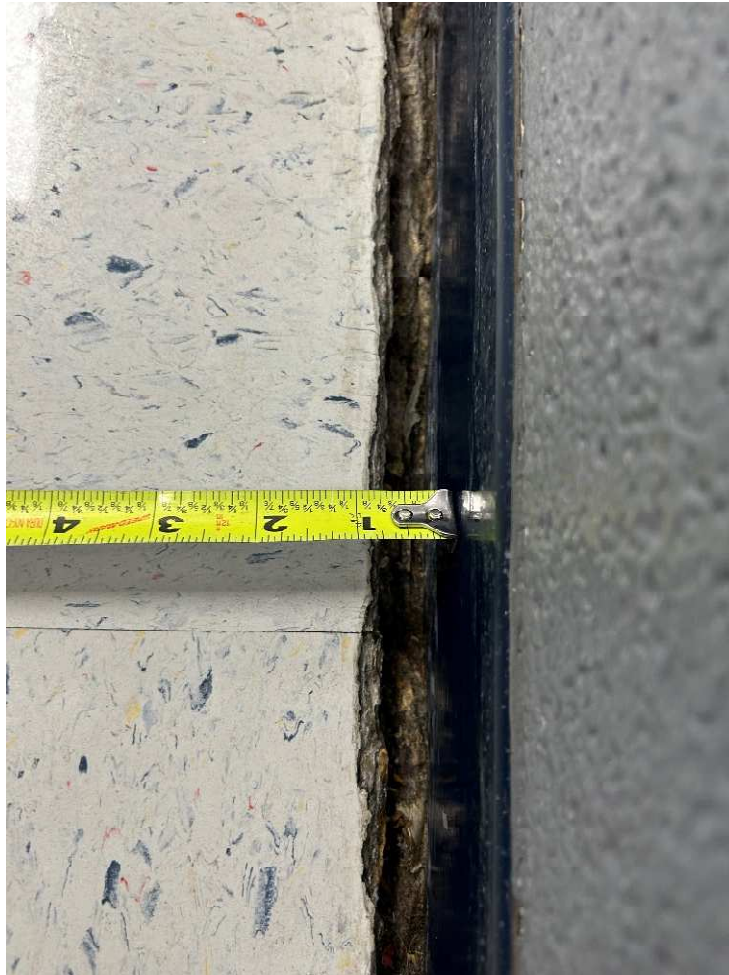
Room 123 shows visible heave.
