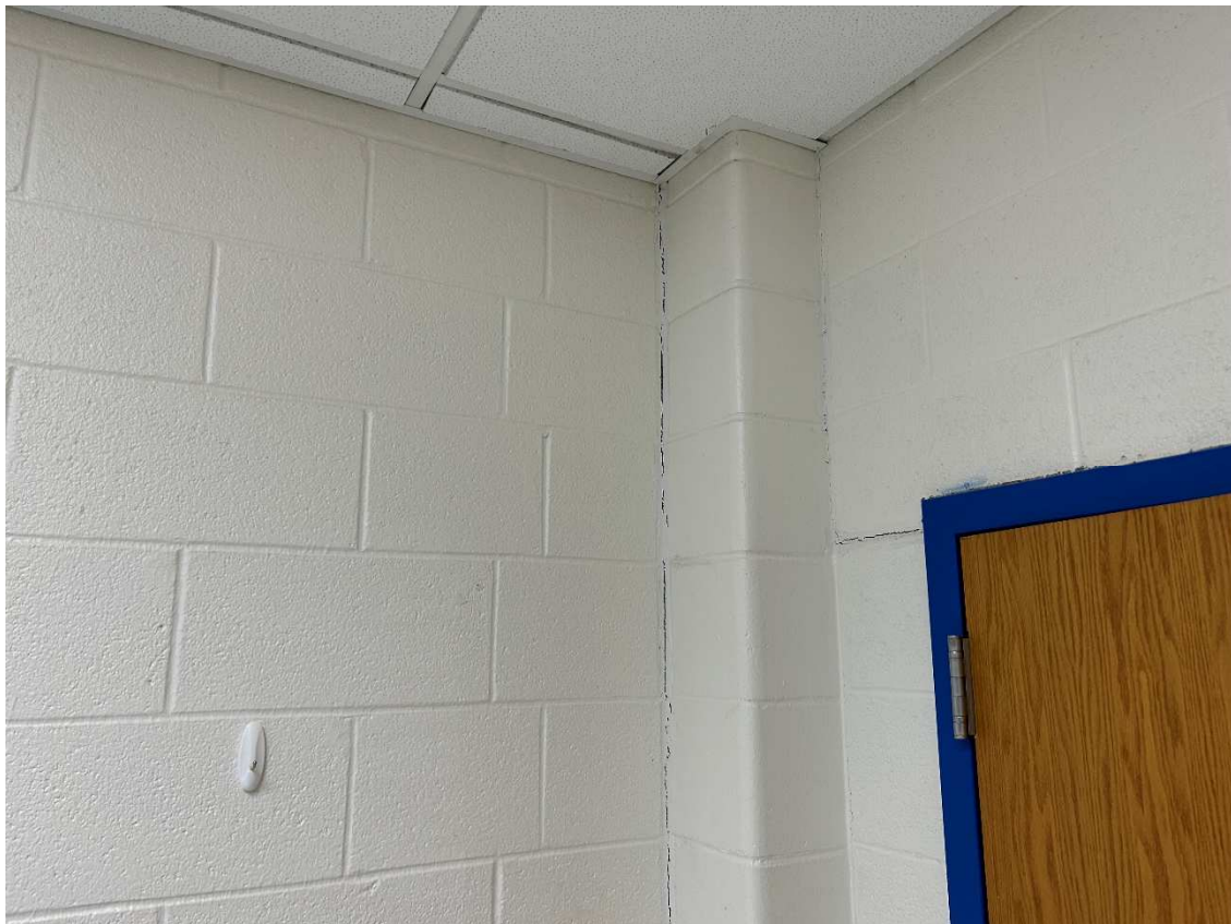
Nurse's office, separation of CMU at wall corner and crack near door.
