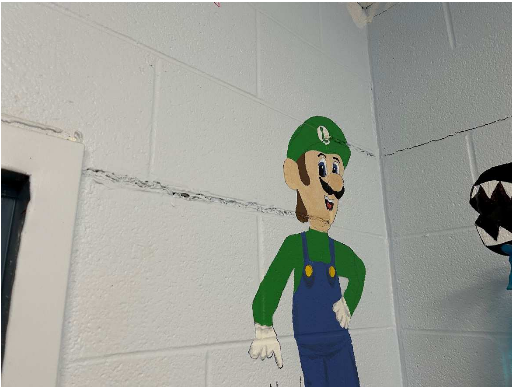
Room 105, CMU cracks in closet area.
