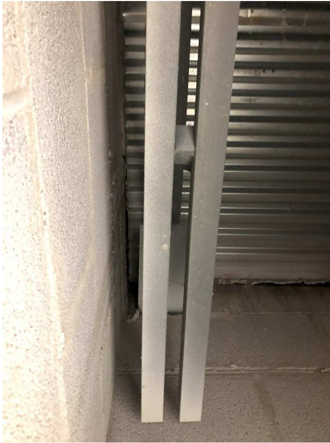
Edge of deck condition at continuous CMU wall (assumed shearwall). No connection to shearwall observed.
