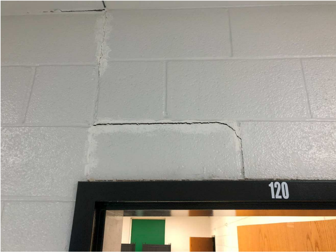
Cracking and deflection of lintel at load bearing wall.
