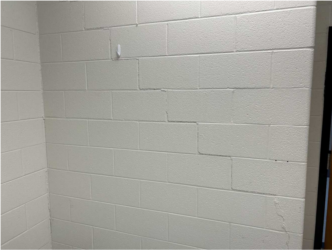
Room 119, with visible cracks in CMU wall.
