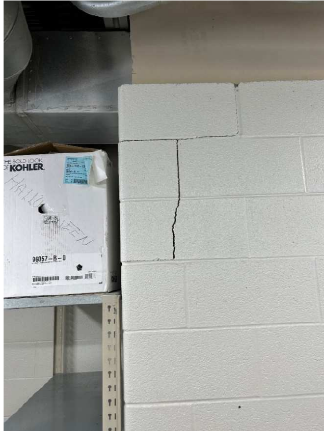
Electrical room (1 st floor) with visible cracks in CMU walls.
