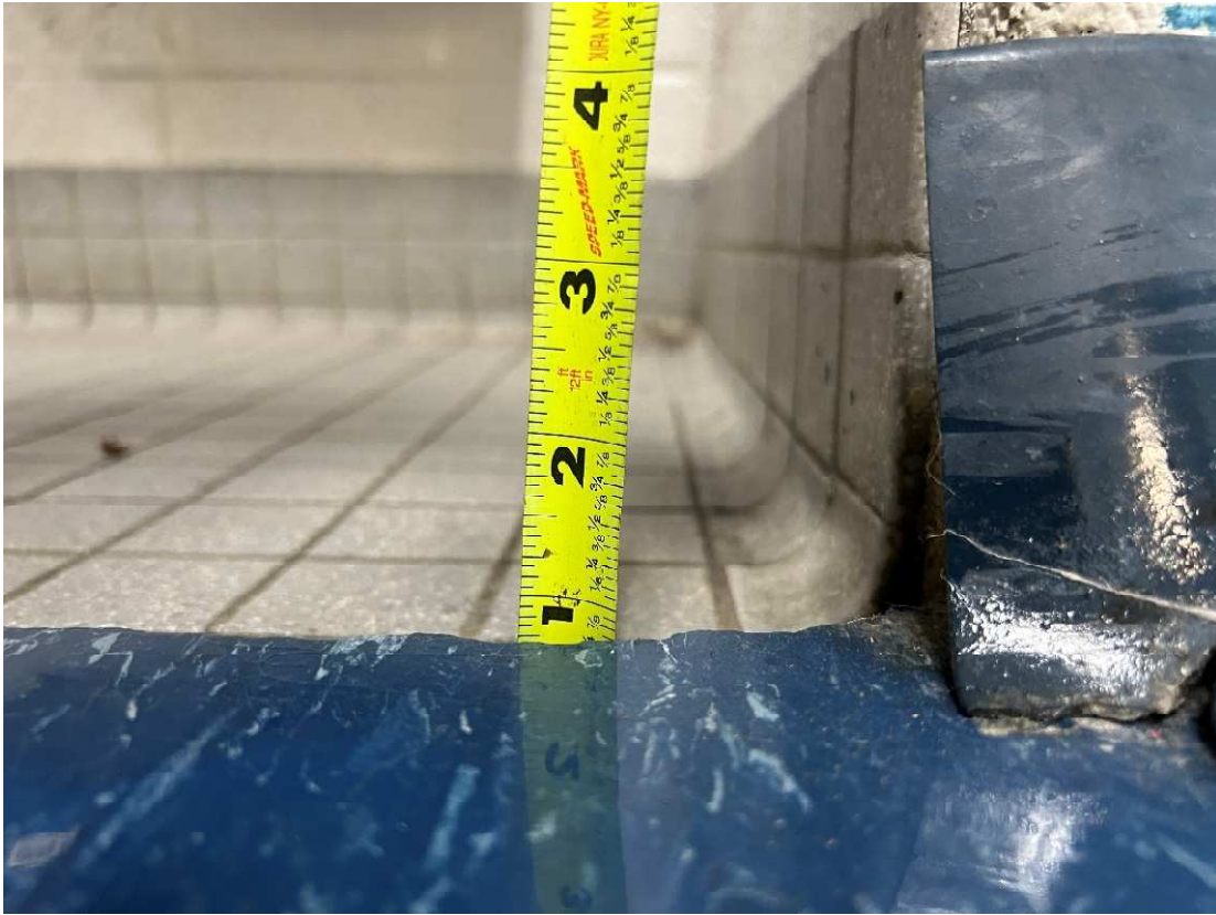
Slab crack at water fountain showing visible heave (3/4" differential).
