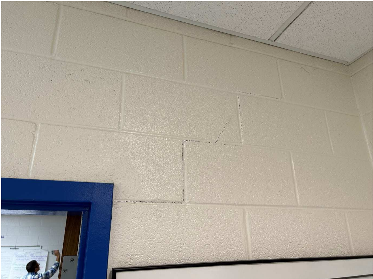
Crack in CMU near youth service center room
