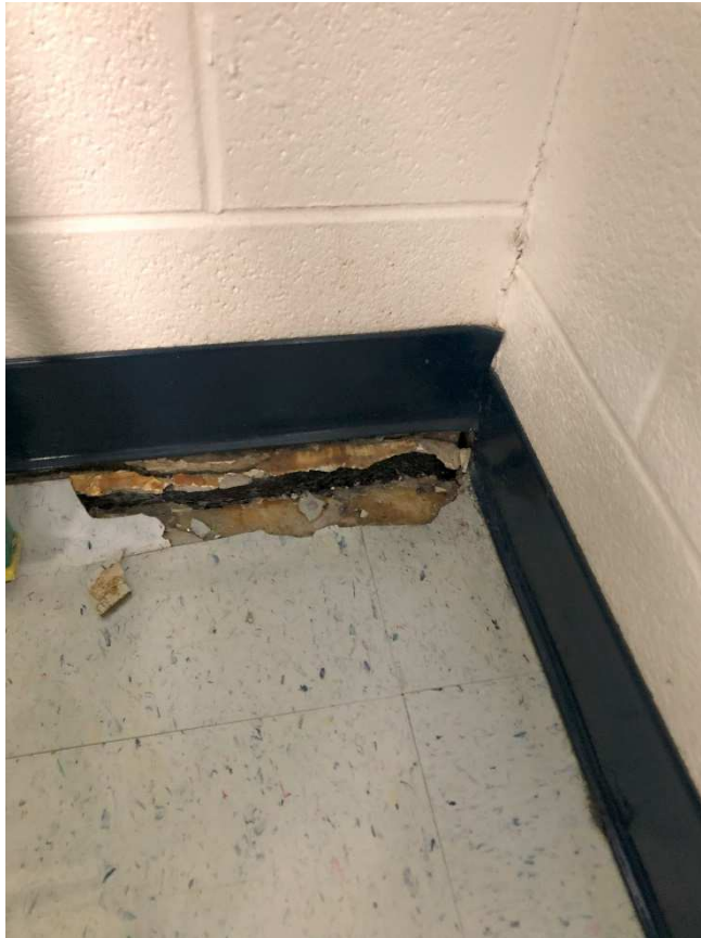
Heaving of continuous CMU @ 2 nd floor level. Suspended concrete slab has not heaved with wall. Some areas appear to have separation of slab from wall, but upon further inspection slab has not significantly separated from CMU wall.
