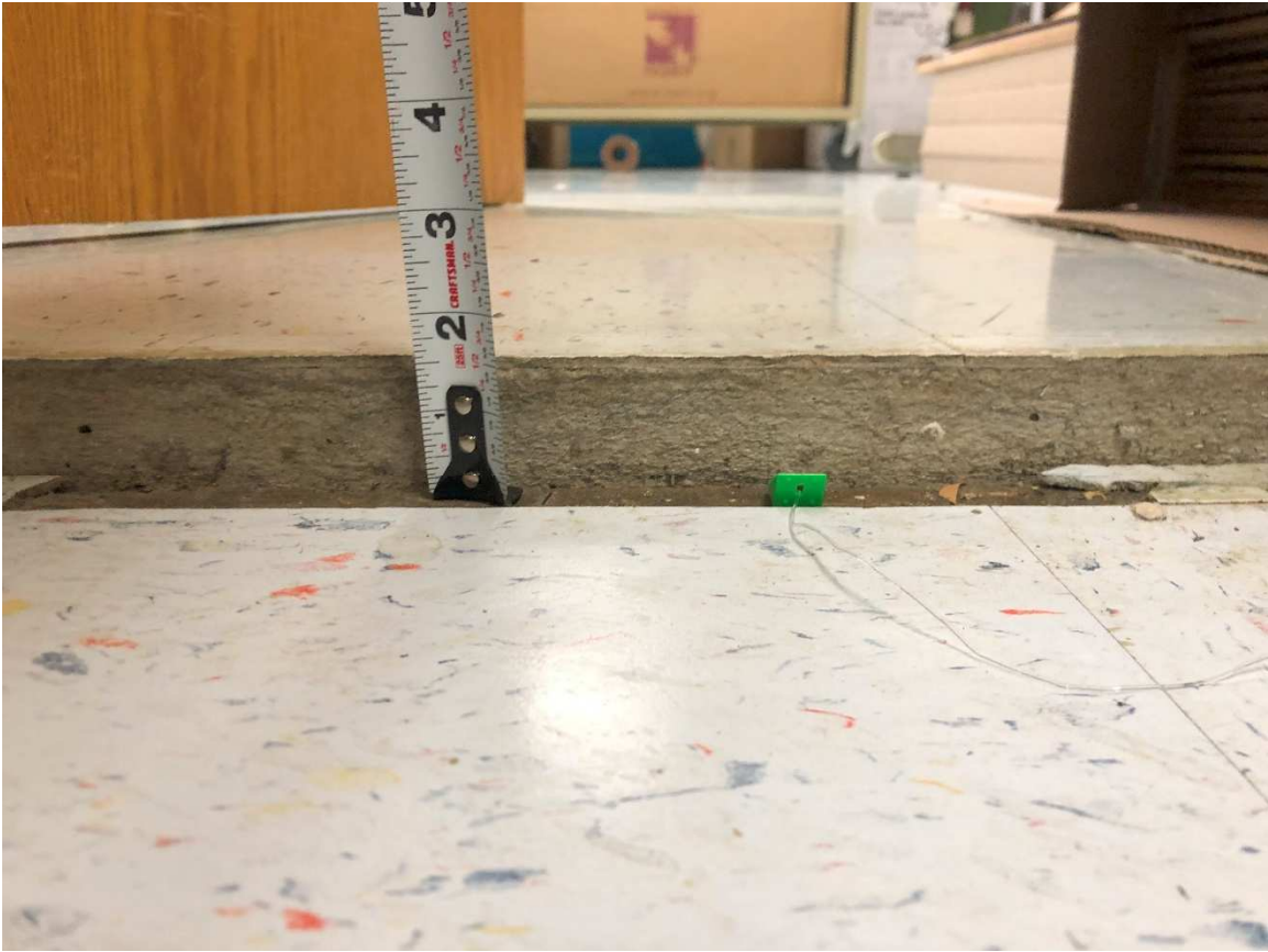
Slab heave @ construction joint
