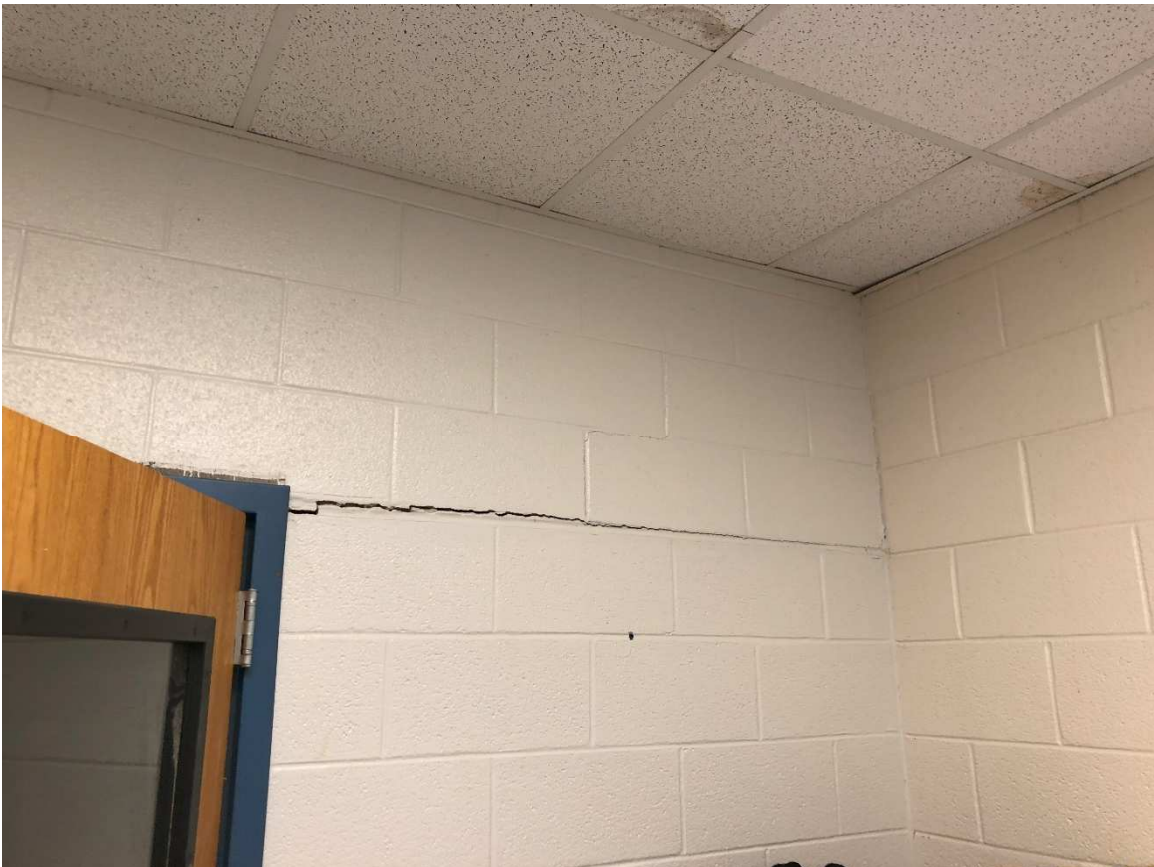
Horizontal crack in CMU
