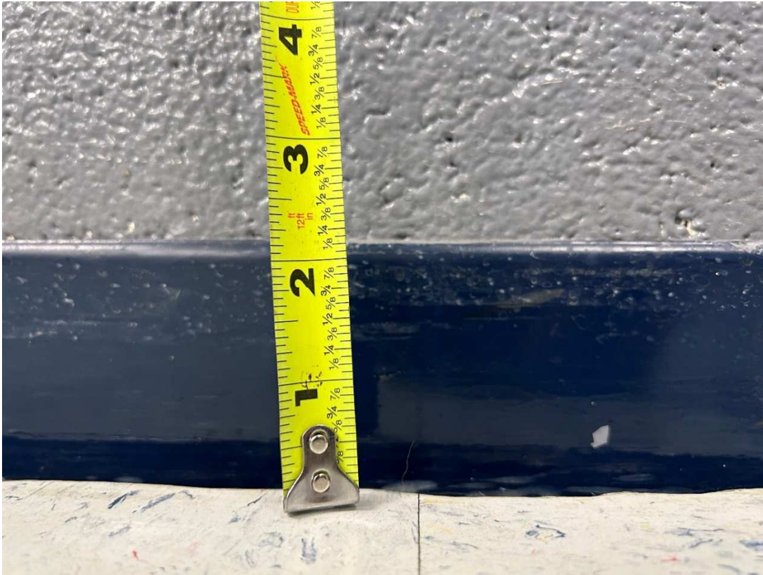
Room 123 showing approx. 2" of heave in areas.
