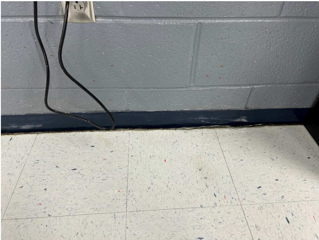
Room 123 showing visible heave in floor slab.
