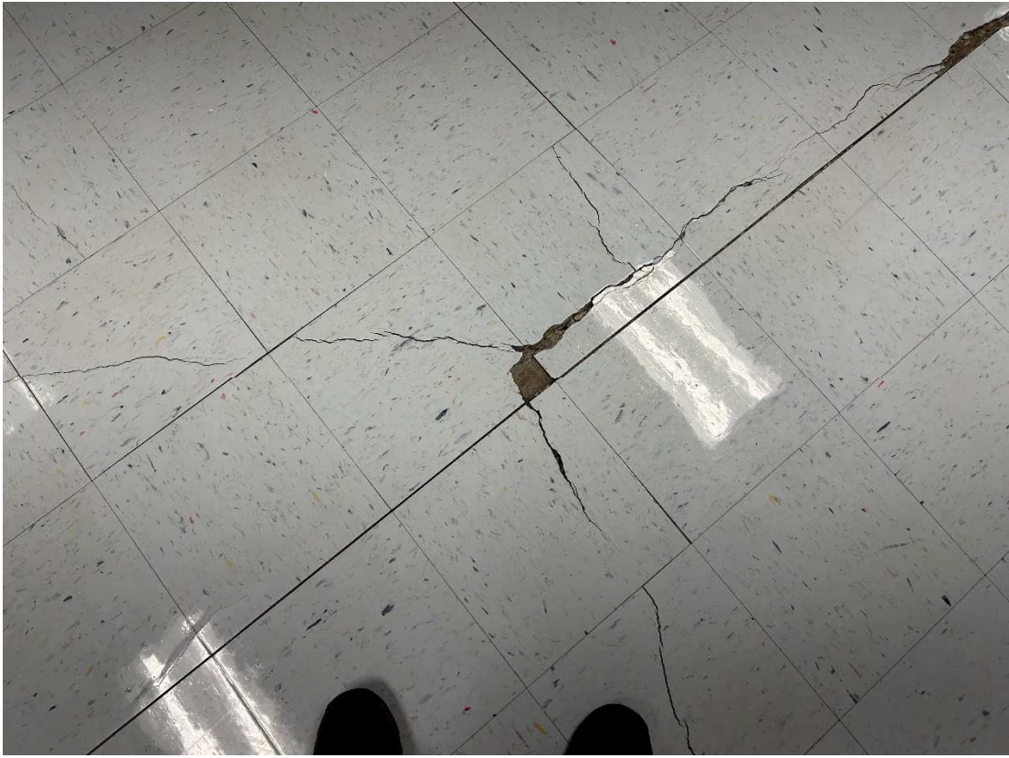
Cracks in slab of hallway
