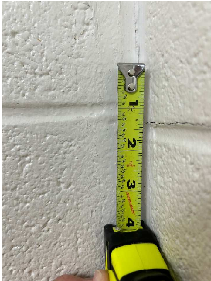
Room 121, CMU coursing showing approx 1/2" heave between exterior and interior walls.
