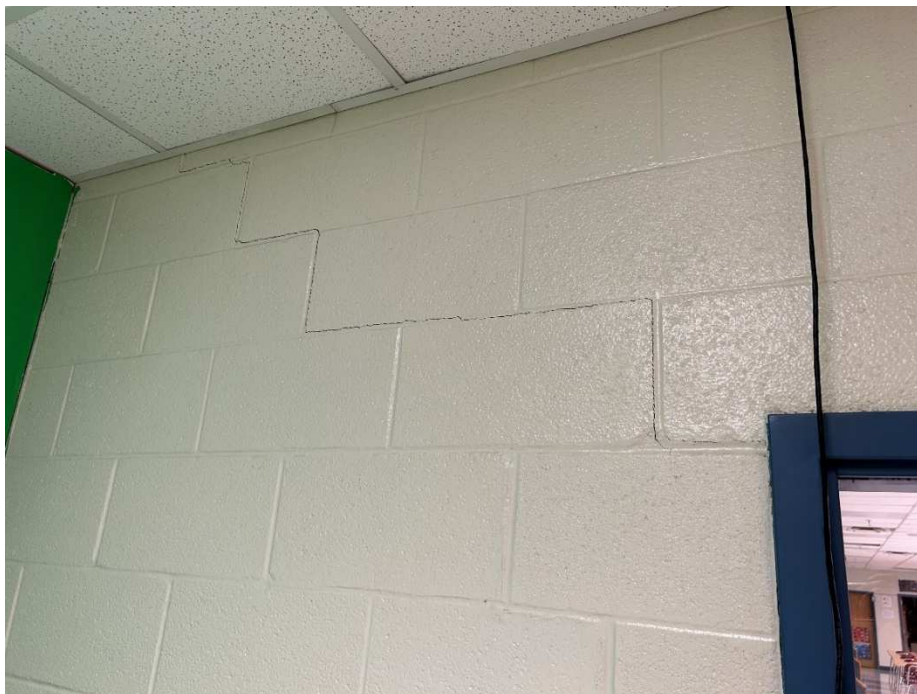
Room 131, cracks in CMU near door of green screen room.
