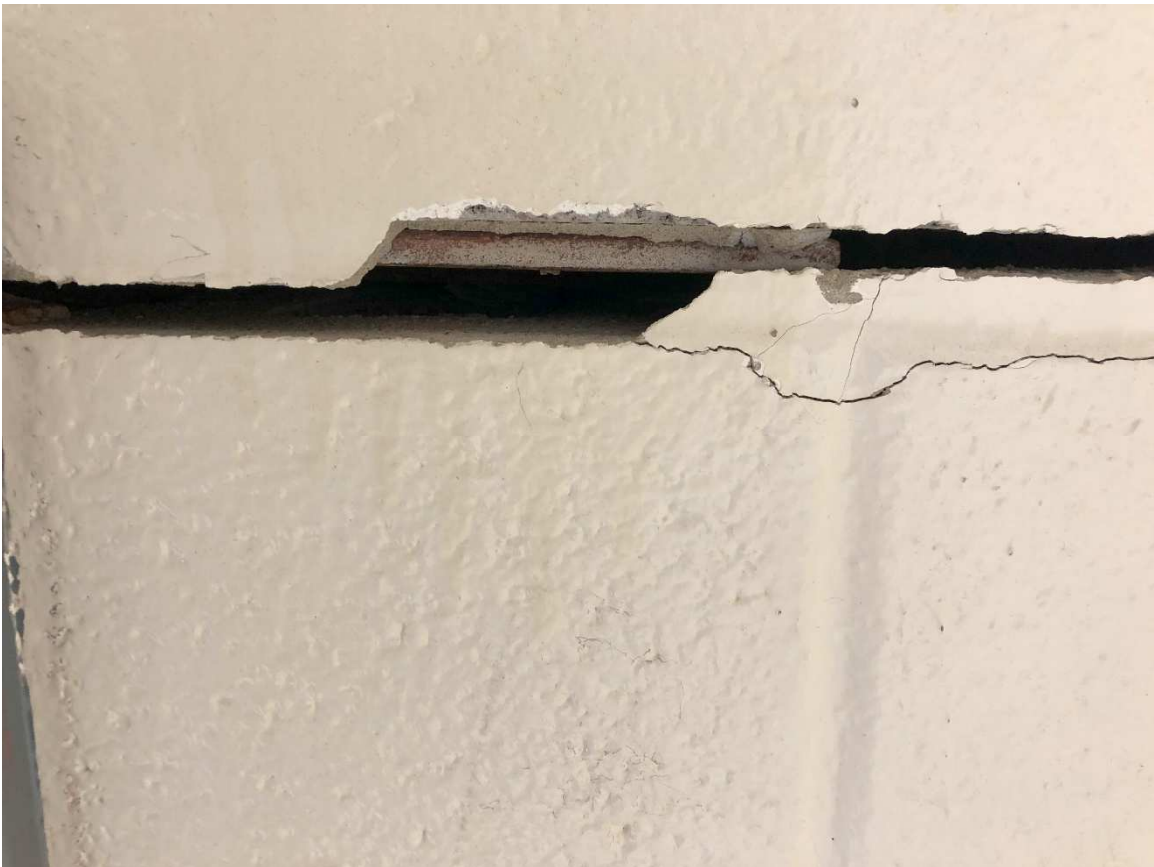
Significant cracking at steel lintel
