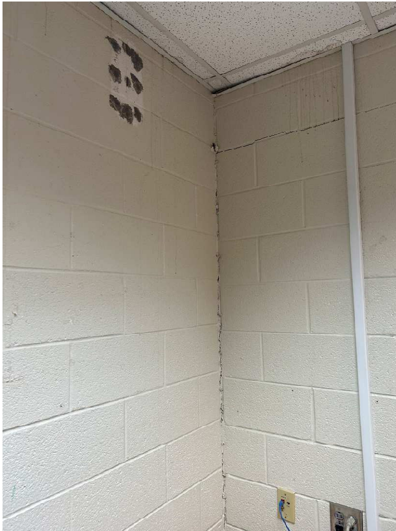
Room 131, cracks in CMU wall with heave visible in coursing.
