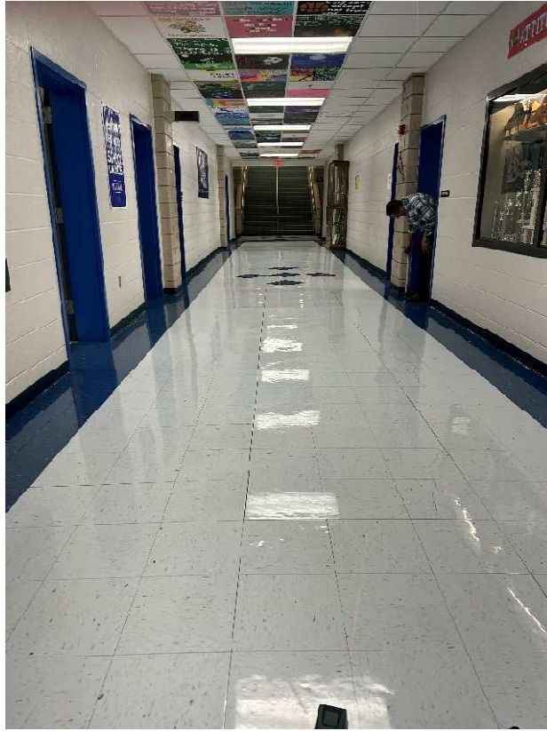
View of hallway w/ slab heave
