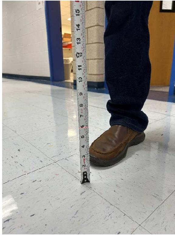
Laser level indicating a rise in concrete slab of approx. 2" from exterior door to mid-point in classroom hallway.
