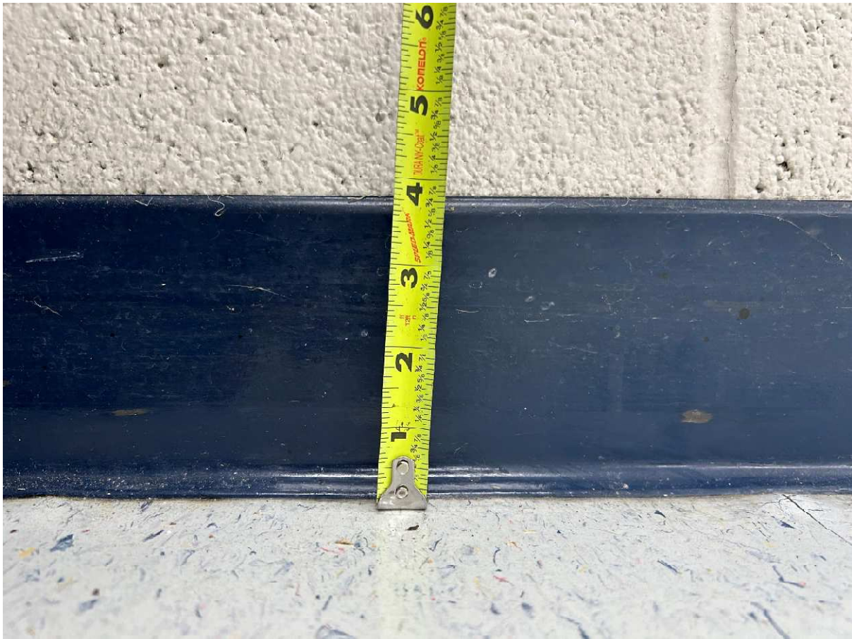
Room 121 at location where vinyl wall base fully visible (no visible heave in slab)
