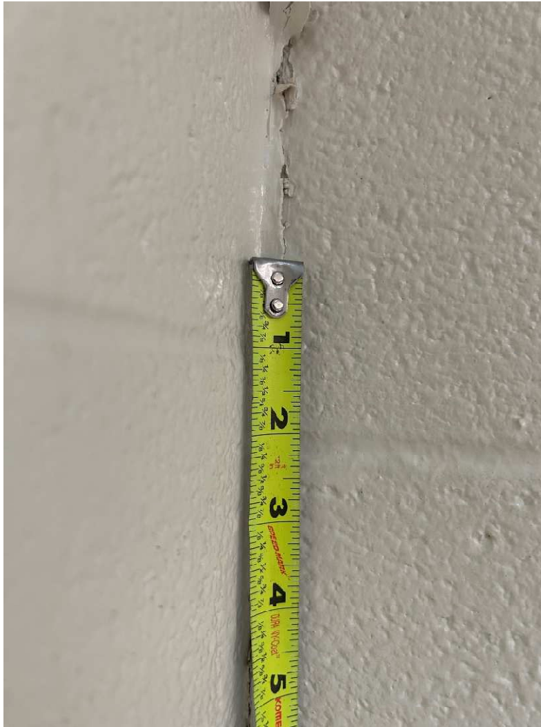
Room 131, showing approx. 1"+ heave between interior and exterior walls.
