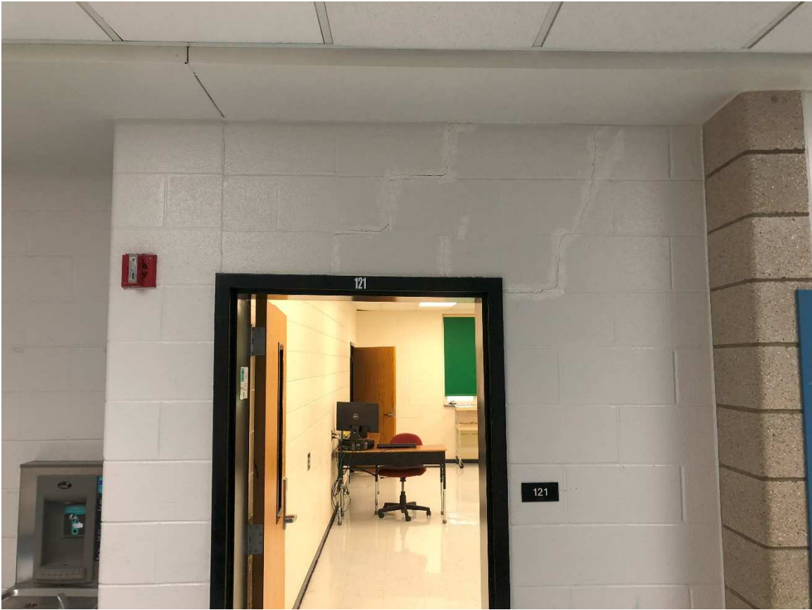
Cracking and deflection of lintel at load bearing wall. Door frame out of square.
