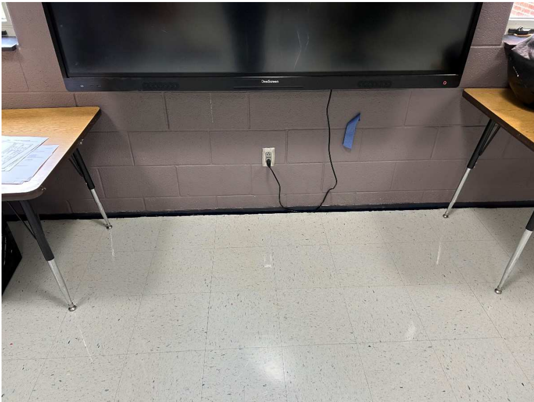
Room 105 slab showing heave in slab, approx. 3"
