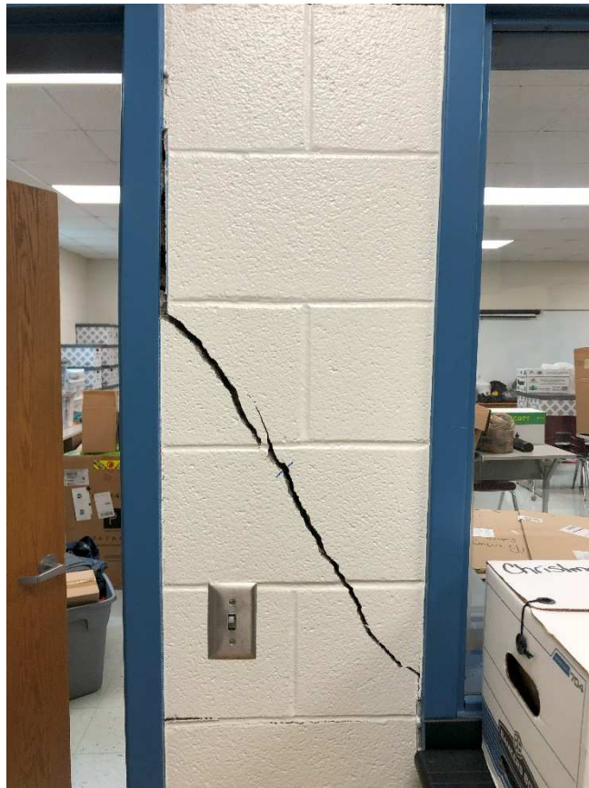
Significant crack in partition wall
