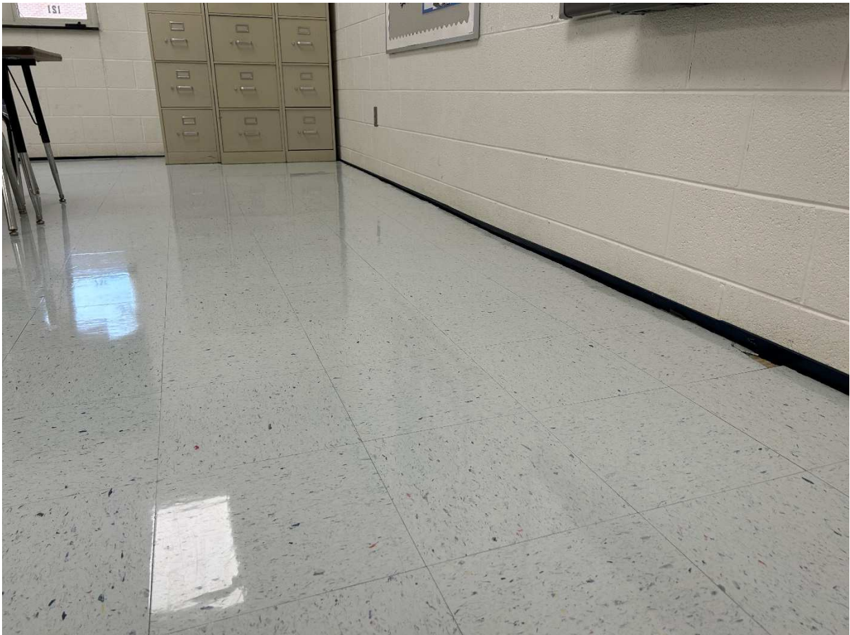
Room 121 showing slab heave. Up to 3 1/2" +/- heave.
