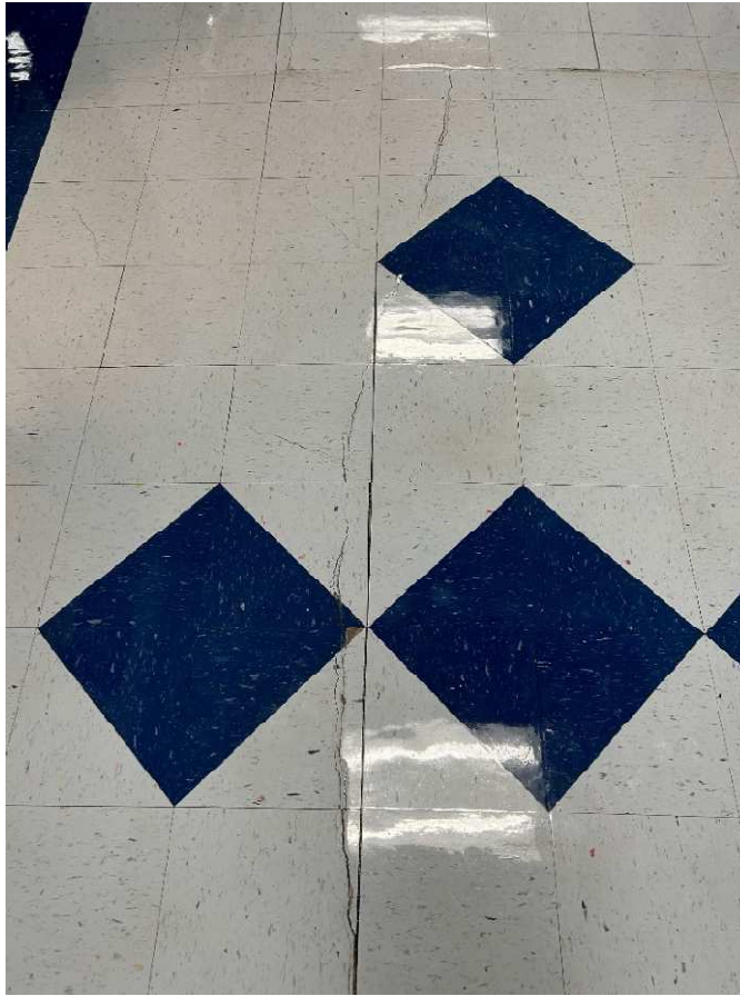
Heaving of slab
