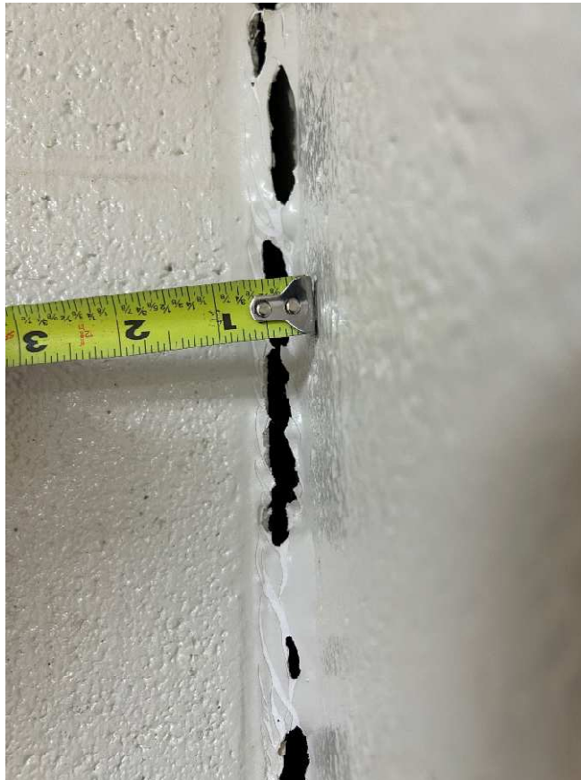
Closeup of Room 131 gap, approx 1/2" wide.
