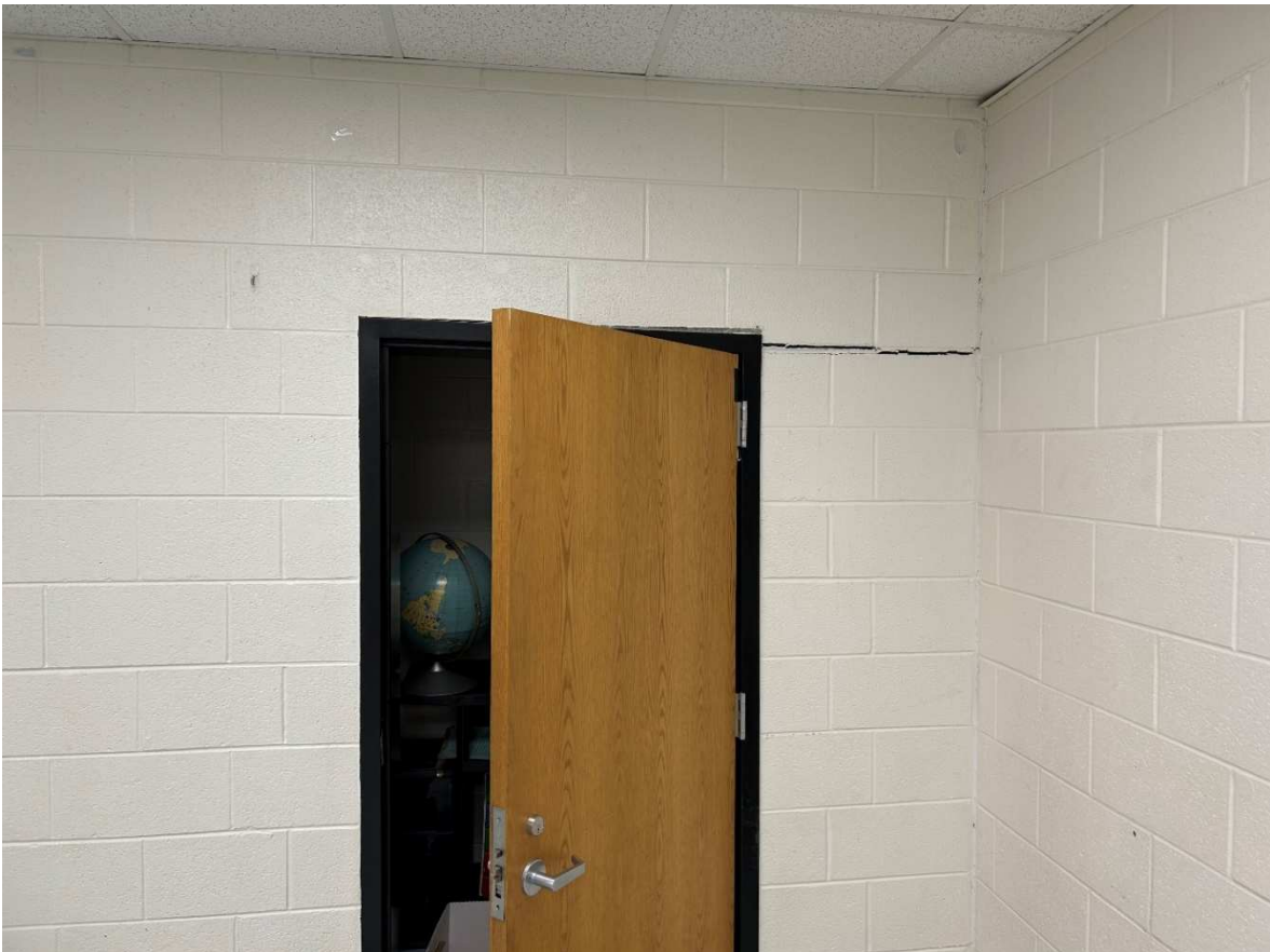
Crack in CMU to the right of closet door. Door frame out of square.
