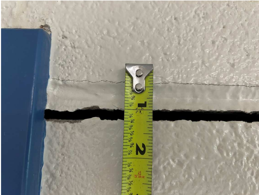
Approx 1/4" gap in CMU course, Room 131
