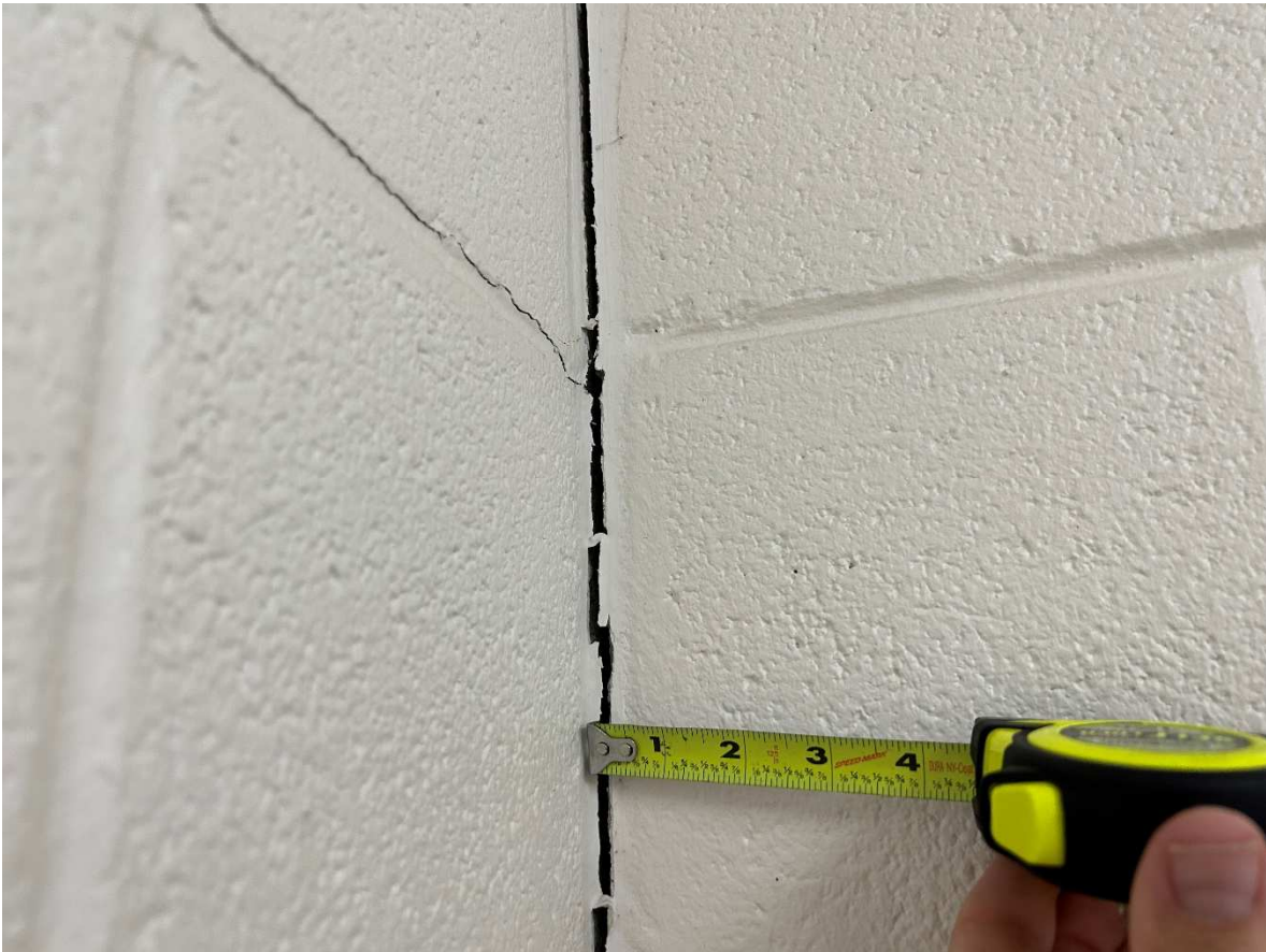
Nurse's office, separation of CMU at wall corner.
