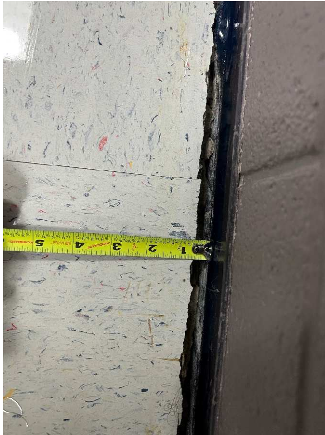
Room 105 slab heaved and showing gap from CMU interior wall.
