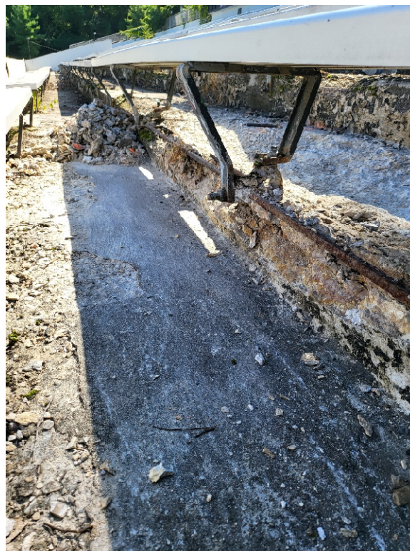
Photo 4: Typical conditions at the lower portion of the stands. Note the rusted reinforcing bar and "chalky" concrete texture indicating significant carbonation in the concrete.
