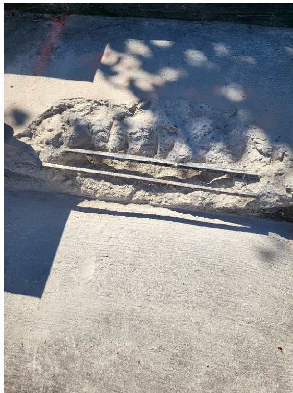
Photo 2: Exposed reinforcing at the top of the stands. The reinforcing was found to be 1/2", square bars with deformations and signs of corrosion or rust. The concrete was also found to be in good condition. This condition is typical at the top of the stands.
