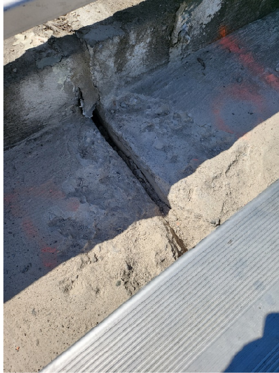
Photo 1: This photo is one of three expansion joints that run from the bottom of the stands to the top. The existing joint material was removed for further observation. These joints will need to be replaced their entire length.
