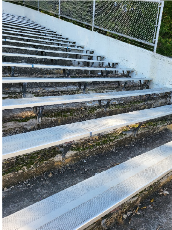
Photo 3: Typical conditions of the lower portion of the stands. This photo was taken at the north of the stands. Note the cracking at the face of each step and the moss growth indicating that this area is subjected to continuous moisture conditions.
