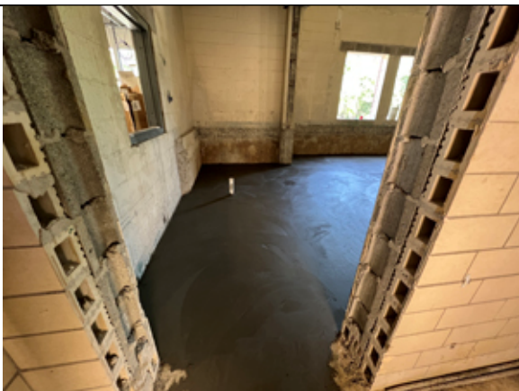
The new concrete floor at the SRO office and Faculty Lounge has been poured.
