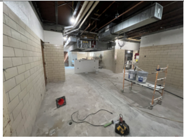
The Kitchen floor is being prepped for installation of the epoxy flooring.
