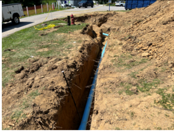
Installation of the water line for the fire vault is being installed.
