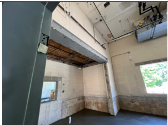
The steel channel lintel has been installed at the wall between the SRO office and Faculty Lounge.
