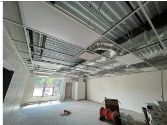
The ceiling grid, lights, and HVAC grilles have been installed in the classrooms of the new addition.
