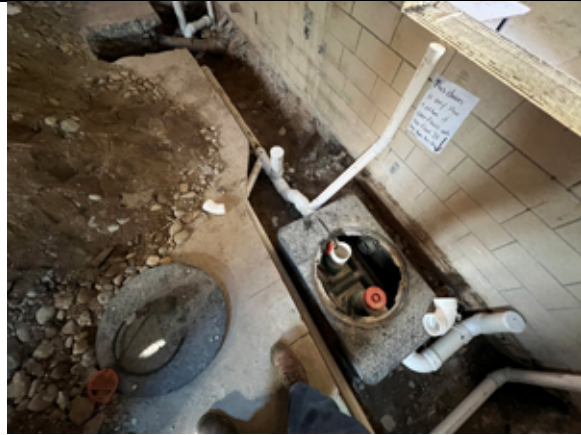
Underslab plumbing for the new equipment is being installed in the kitchen.
