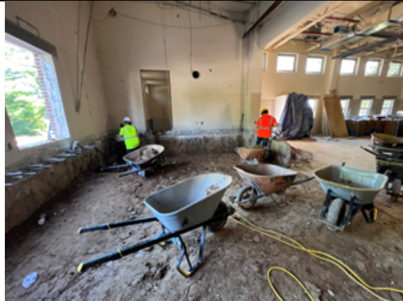
The stage slab has been removed. Workers were excavating excess soil to permit installation of the new floor slab.
