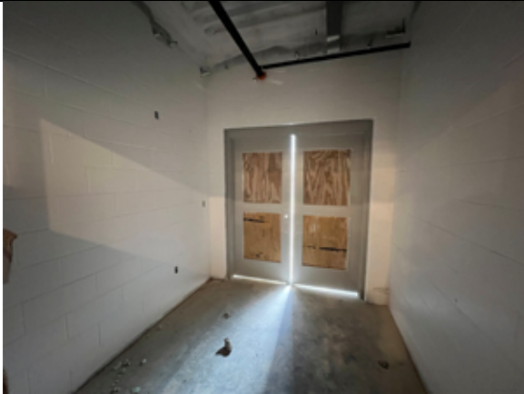
The new hollow metal doors have been installed in the new addition.
