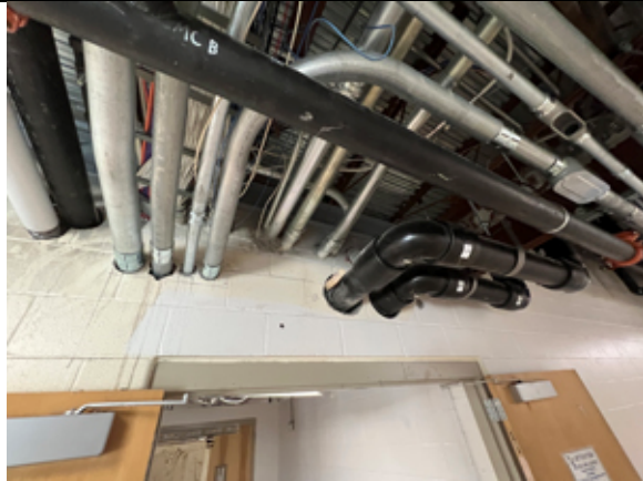
The steel reinforcing channel has been installed above the MEP penetrations as the connection between the original building and previous addition.
