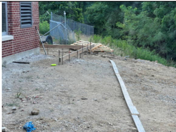
Formwork is being installed for the walks outside the new Pre-K classrooms.
