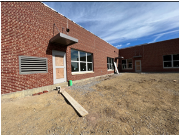
The brick on the new addition has been cleaned and the control joints caulked.
