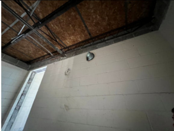
The wall between the new SRO's office and new faculty lounge was determined to be a bearing wall.
