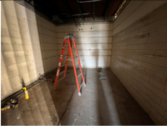
The existing walk-in cooler has been removed. No VAT was under the cooler.
