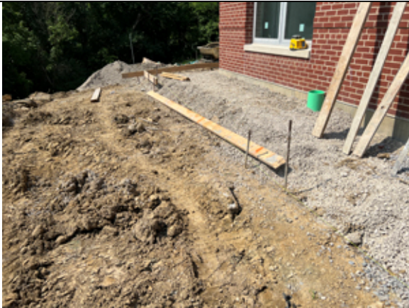
Installation of the new concrete paving at Pre-K classrooms is in progress.
