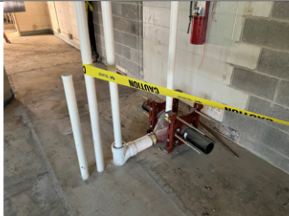
Carriers have been set for the new toilets in the Admin Suite.
