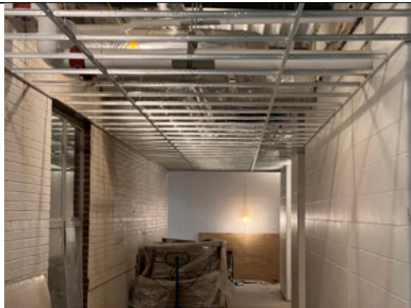
The ceiling grid has been installed in the corridor of the new addition.
