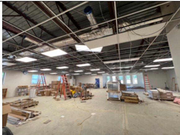
A view of the Media Center with the grid and light fixtures installed.
