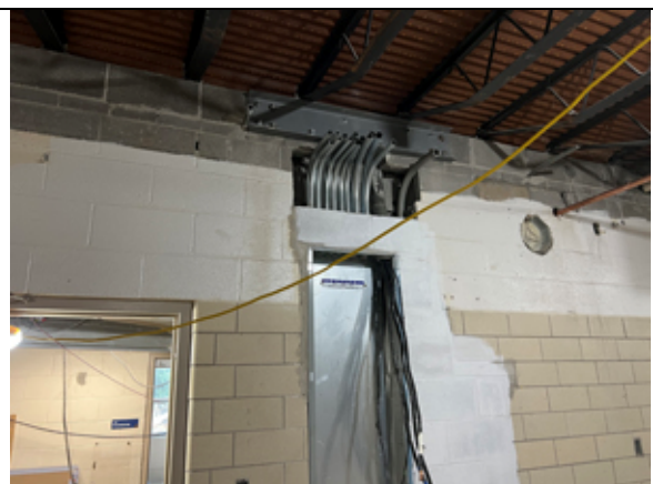
The steel reinforcing channel has been installed over the new electric panel.
