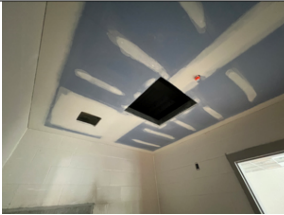
The gypsum board ceiling has been installed in the toilet rooms of the new addition.
