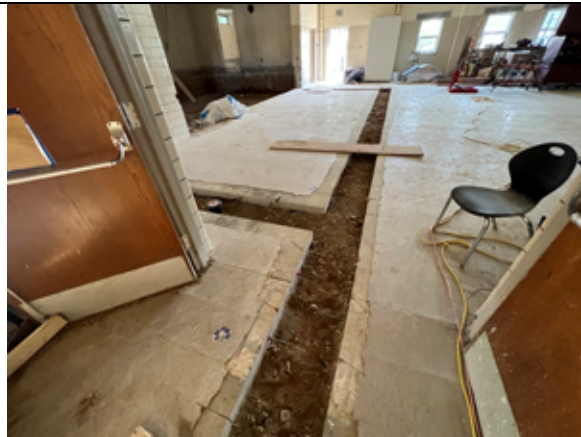
The floor slab for the new plumbing from the Faculty Lounge has been cut and the plumbing installed.
