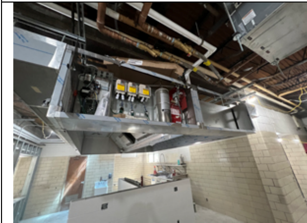
The Ansul system for the kitchen hood.
