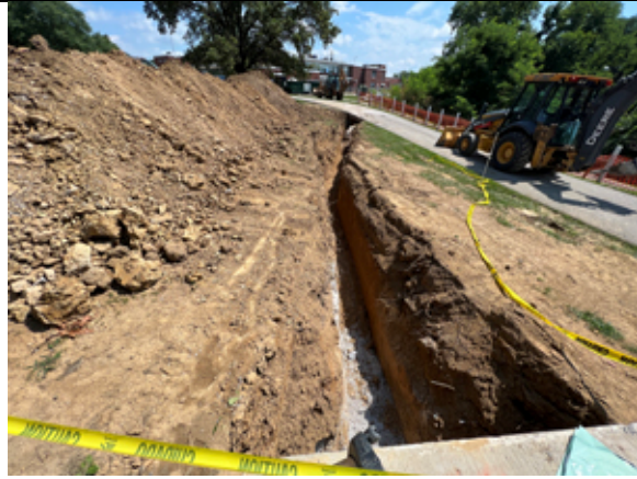
Installation of the water line for the fire vault is being installed.
