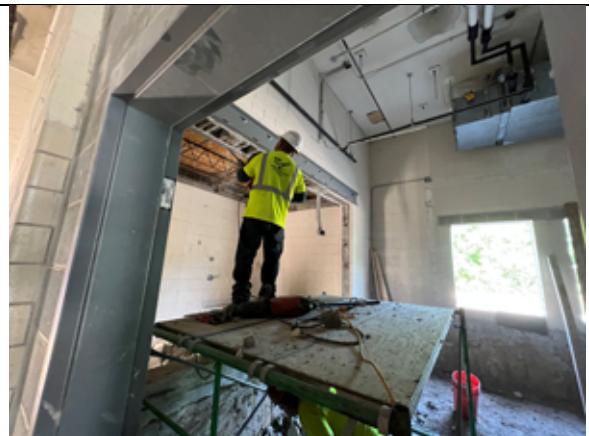
View of new reinforcing channel installed between the SRO office and Faculty Lounge.
