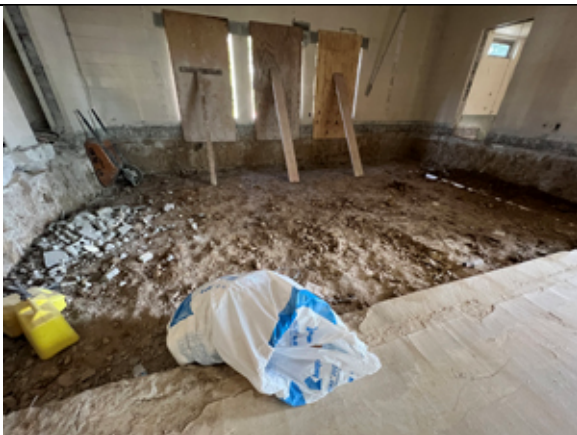
The existing stage removal has been completed and excavated down to the subgrade.
