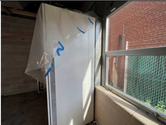
The new HVAC units have been set up against the exterior window wall.
