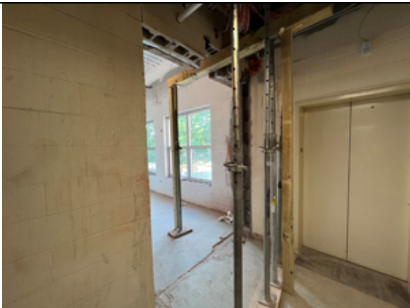
The opening connection between the new addition and existing building at the elevator has been expanded.
