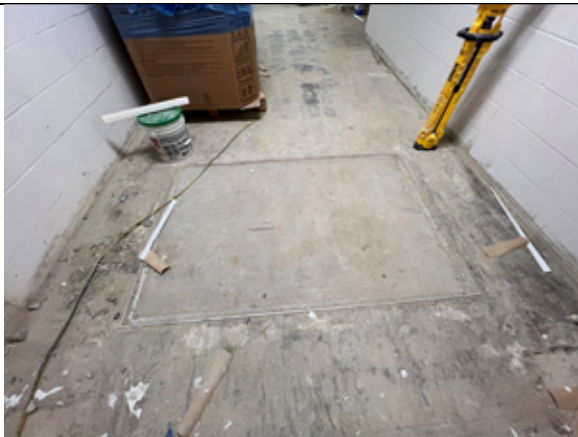
The existing frames for the recessed mats in the original building will be removed and the depression infilled with concrete patching compound.
