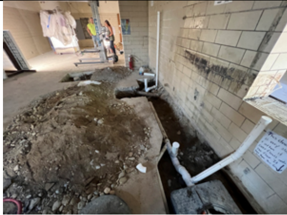
Underslab plumbing for the new equipment is being installed in the kitchen.
