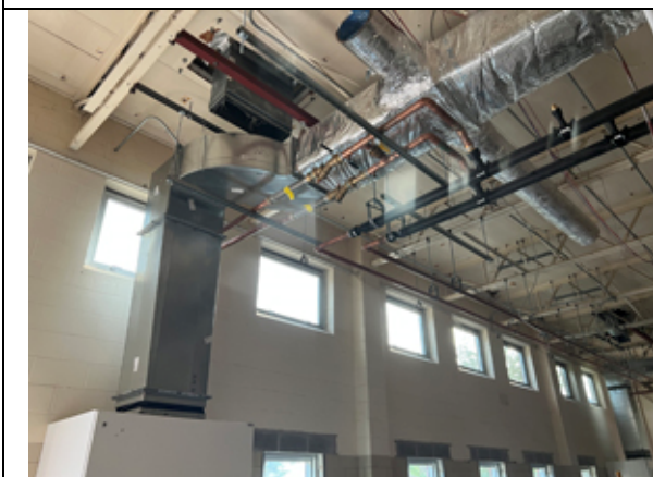
MEP connections are being made to the new HVAC units in the Cafeteria.
