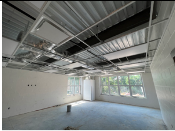
The ceiling grid, lights, and HVAC grilles have been installed in the classrooms of the new addition.
