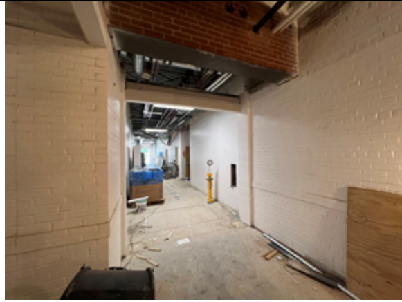
The connection between the existing building and new addition has been completed.
