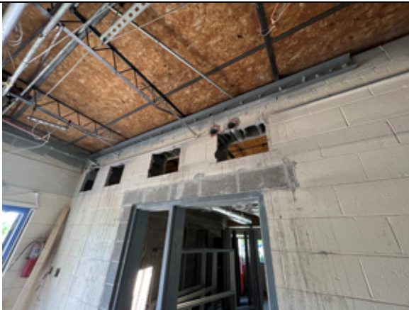
The steel channel reinforcing has been installed over the new MEP penetrations.
