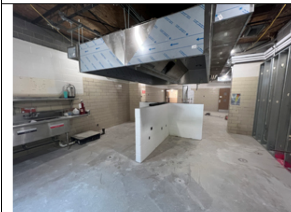
The Kitchen floor is being prepped for installation of the epoxy flooring.
