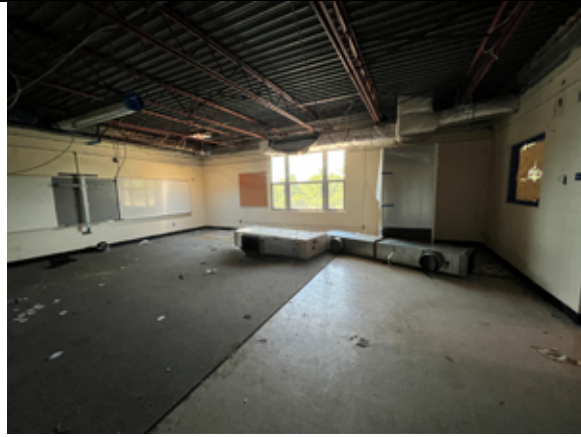
Removal of the existing HVAC equipment is in progress on the second floor.
