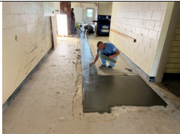
The concrete floors are being patched where the new underslab plumbing was installed.
