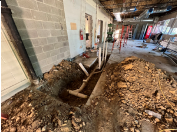
Installation of underslab plumbing in the Admin suite for the new toilet rooms.
