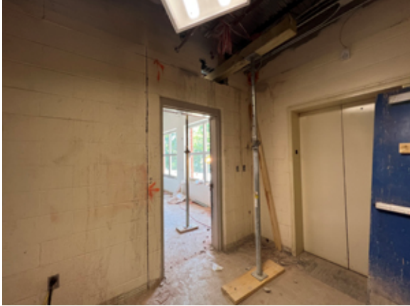
The opening connection between the existing building and new addition is in progress.
