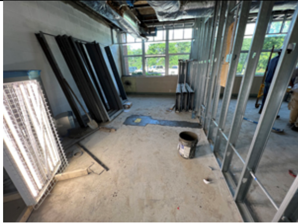
Recessed floor outlet for the Admin Suite Conference Room has been set and the concrete patched.
