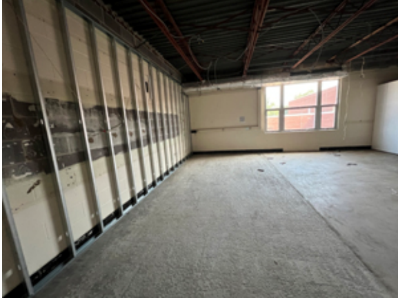
Installation of the stud framing for the presentation walls has been completed.
