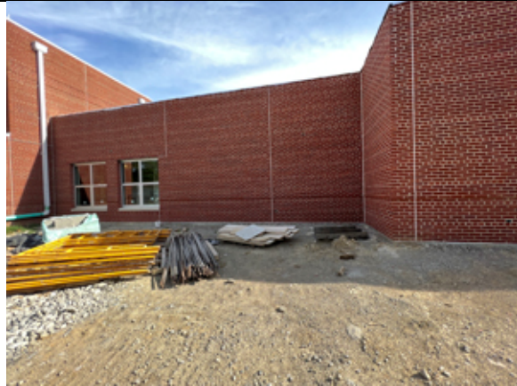
The brick on the new addition has been cleaned and the control joints caulked.
