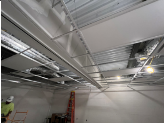
The gypsum board partition has been installed above the folding partition track in the Resource Rooms.
