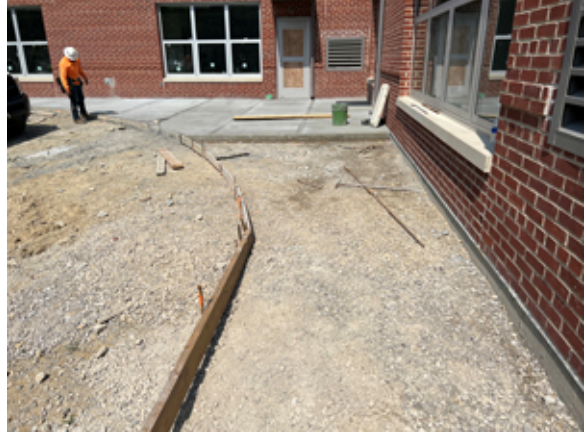
Installation of the new concrete paving at Pre-K classrooms is in progress.
