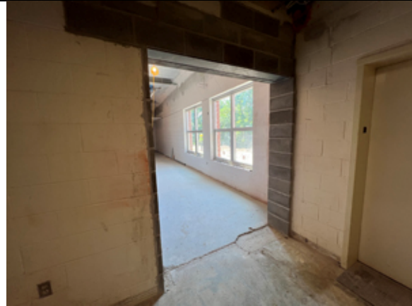
The connection between the existing building and new addition has been completed.
