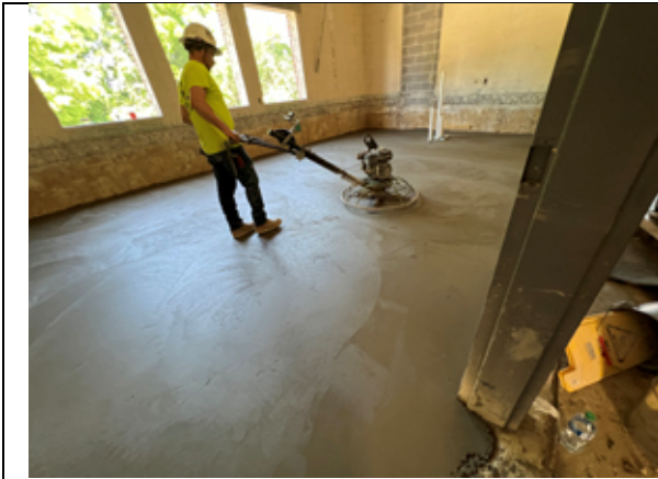
The new concrete floor at the SRO office and Faculty Lounge has been poured.
