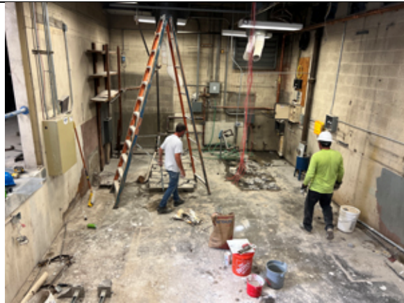
View inside the old mechanical room that is being cleaned out for the new equipment.
