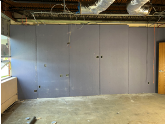
Gypsum board is being installed on the presentation walls in the classrooms.
