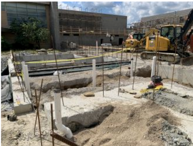
2022.07.13 – Pool equipment room
