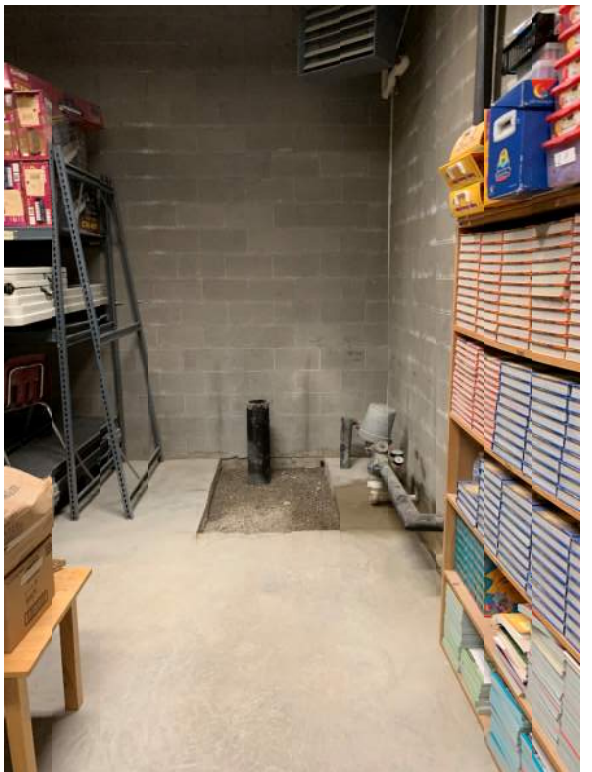
New sprinkler service stub-up
