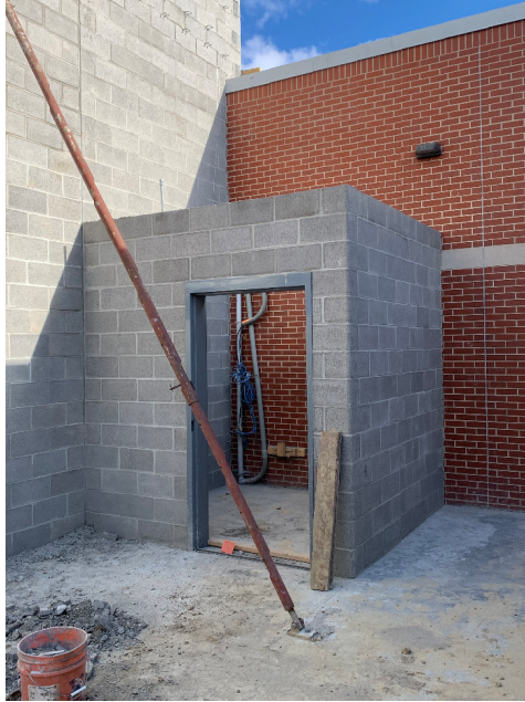
Elevator equipment room
