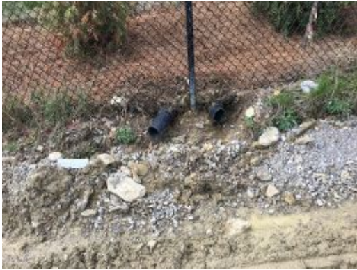
2017.03.30 – Neighbor's downspout collectors discharging onto school property.
