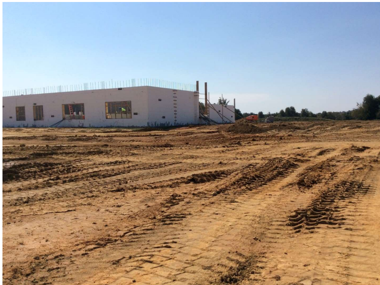
Photo 3: ICF walls now reach the second floor height at the west classroom wing.
