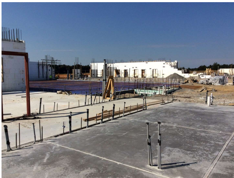
Photo 7: Below slab electrical and plumbing work is complete at the east classroom wing. Concrete slabs have been placed and hollow metal frames are being set in preparation of commencing ICF corridor walls.
