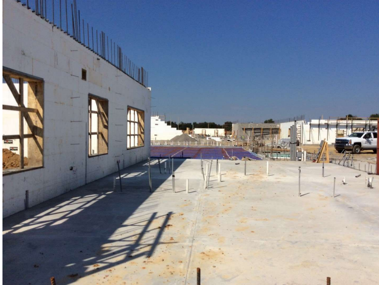
Photo 6: Concrete slab has been placed (foreground). Vapor barrier and slab reinforcement have been placed (beyond) at Gymnasium.
