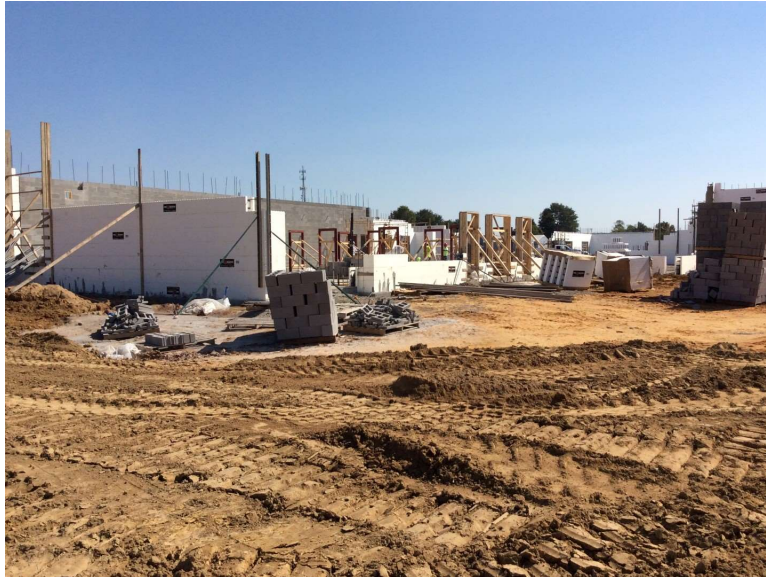
Photo 4: ICF continue at the gymnasium and cafeteria. Masonry (CMU) walls have been laid to service platform elevation.
